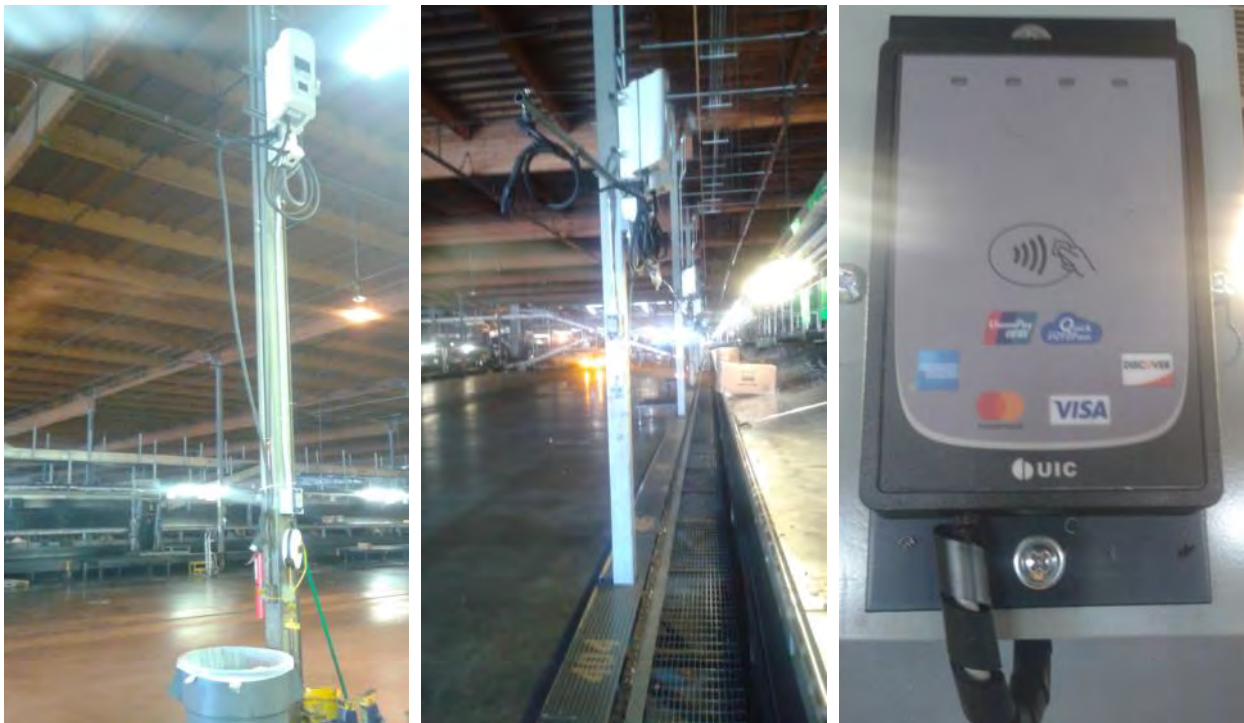
Figure 19. UPS custom overhead EVSE installation, with a variety of charge session activation options
