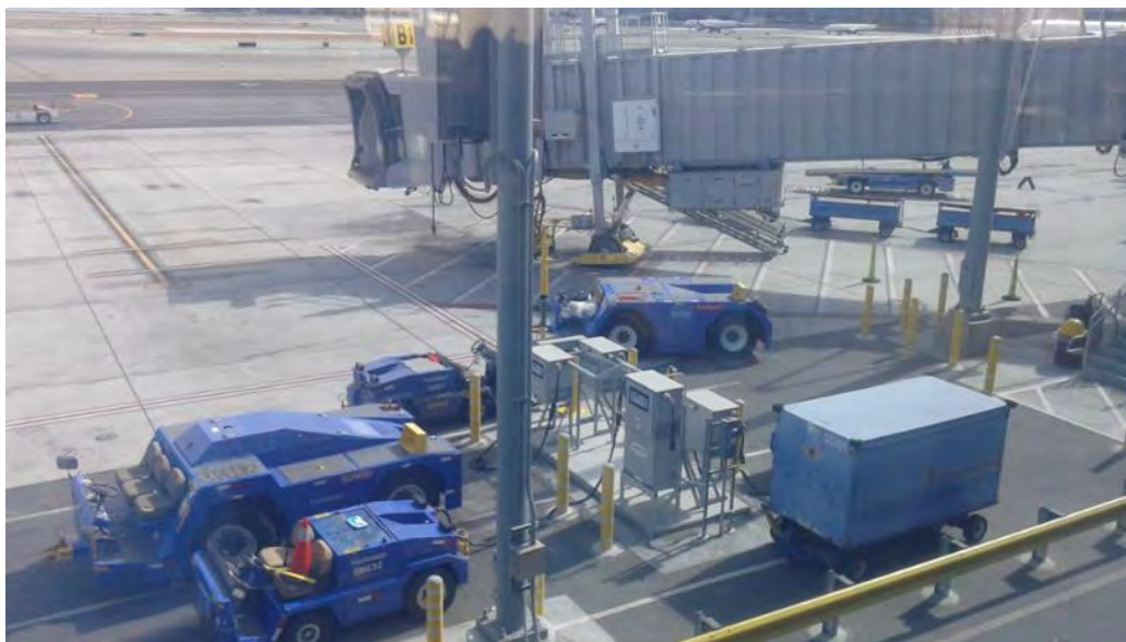
Figure 51. A variety of available electric GSE charging at a California airport
