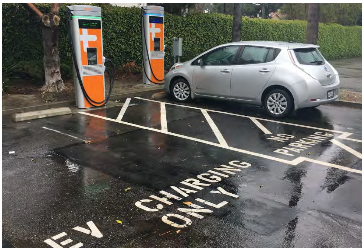
Figure 188. AAA site in Artesia with two DCFCs installed
