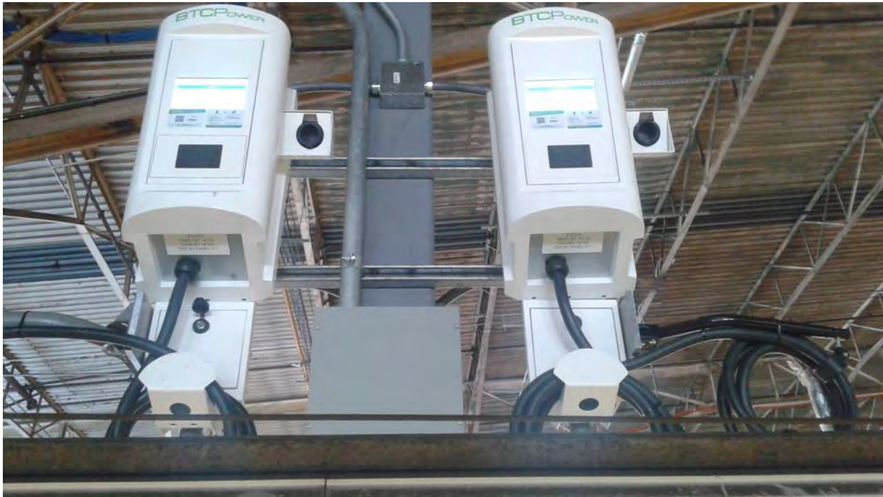
Figure 18. UPS BTC Power L2 EVSE from Greenlots
