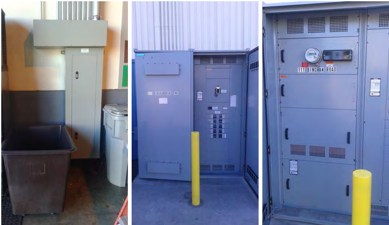
Figure 21. UPS San Marcos EVSE supporting infrastructure
