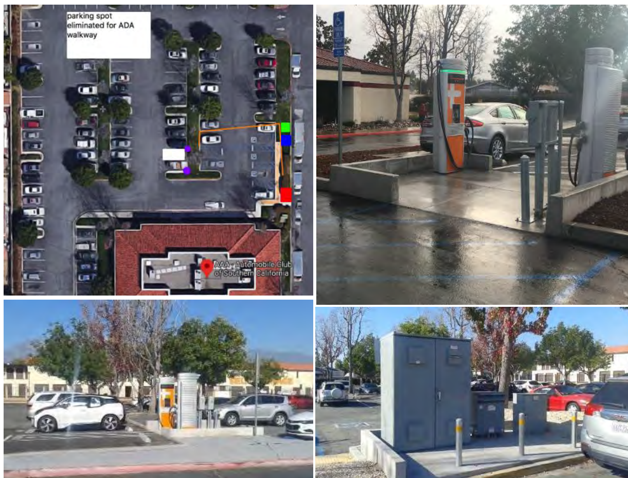
Figure 187. AAA DCFC installation in Upland
