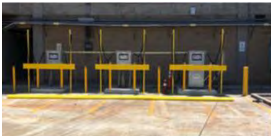
Figure 53. Three installed chargers
