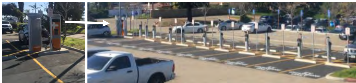
Figure 90. Row of chargers, with DCFCs at one end where better positioning could have increased access by four parking spaces
