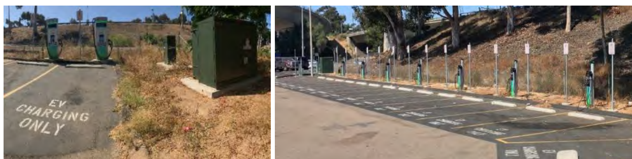
Figure 92. DCFCs on dedicated parking spaces and dual-port L2 stations between parking spaces with signage at each space
