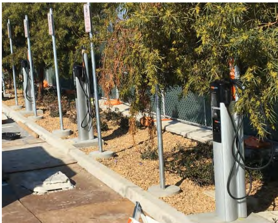
Figure 94. One of the L2 EVSE rows at Chula Vista
