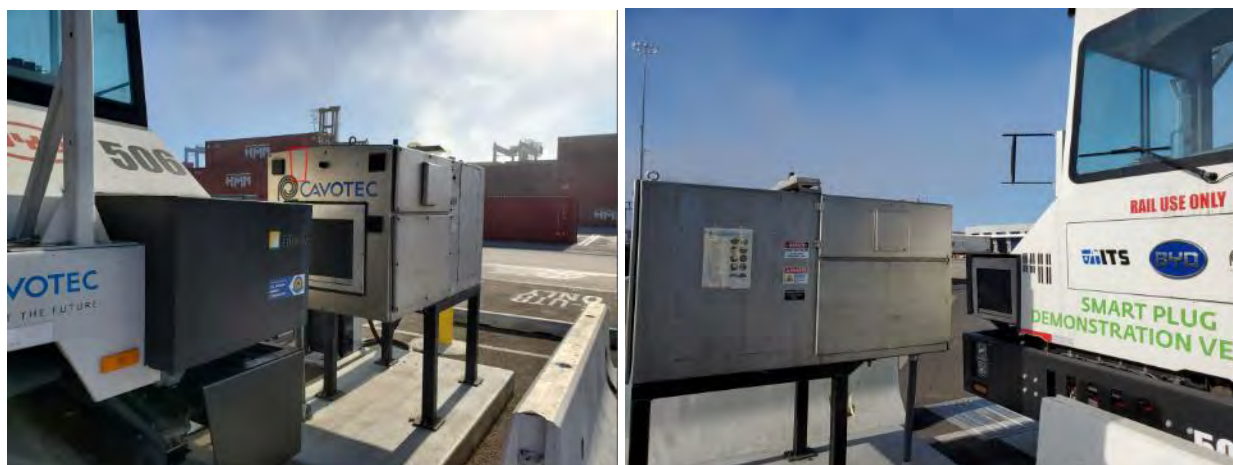
Figure 134. Cavotec automated yard tractor charger
