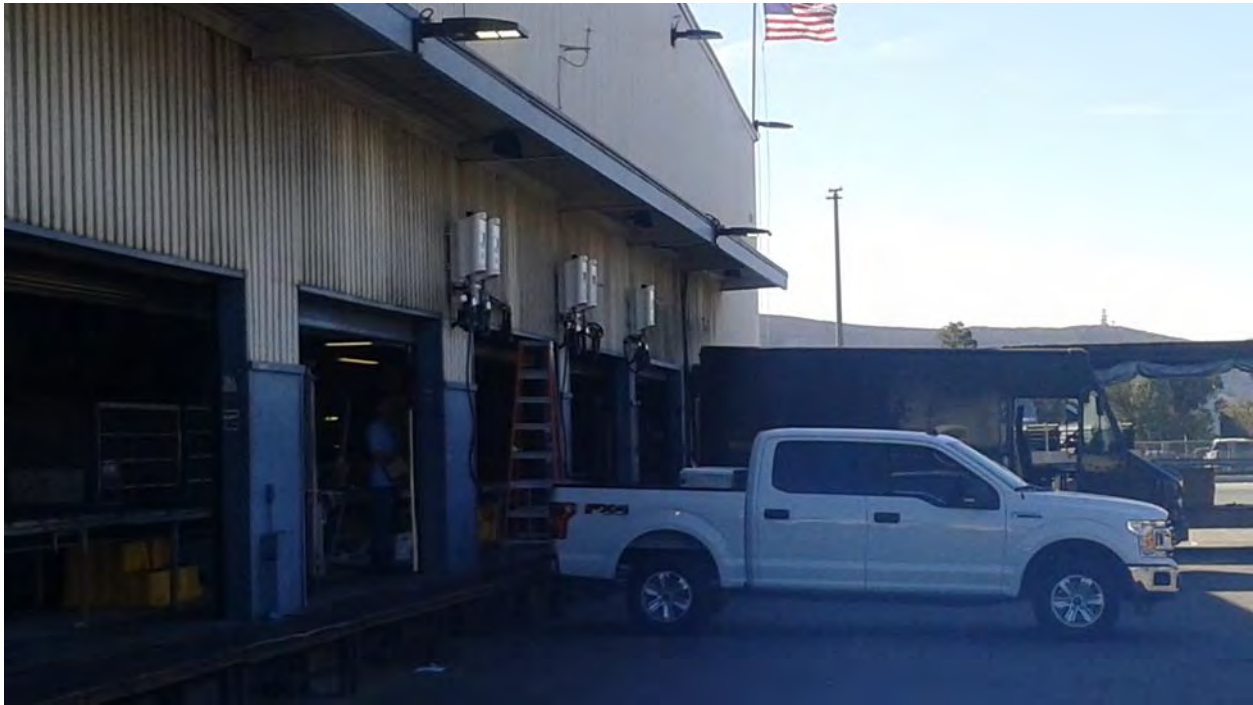
Figure 20. UPS San Marcos overhead EVSE installation
