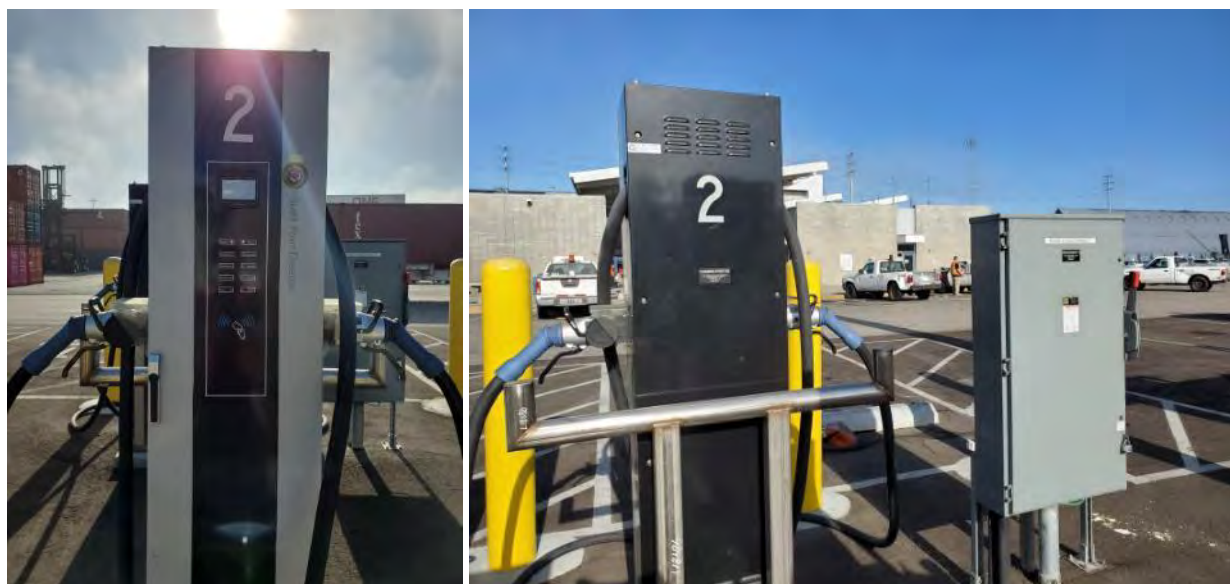
Figure 135. One of six BYD yard tractor chargers
