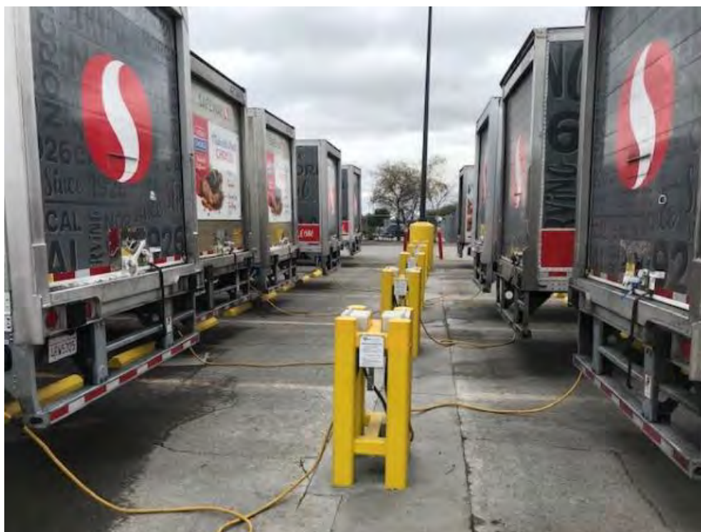
Figure 239. SafeConnect ports in use at staging area, with protective mounting system
