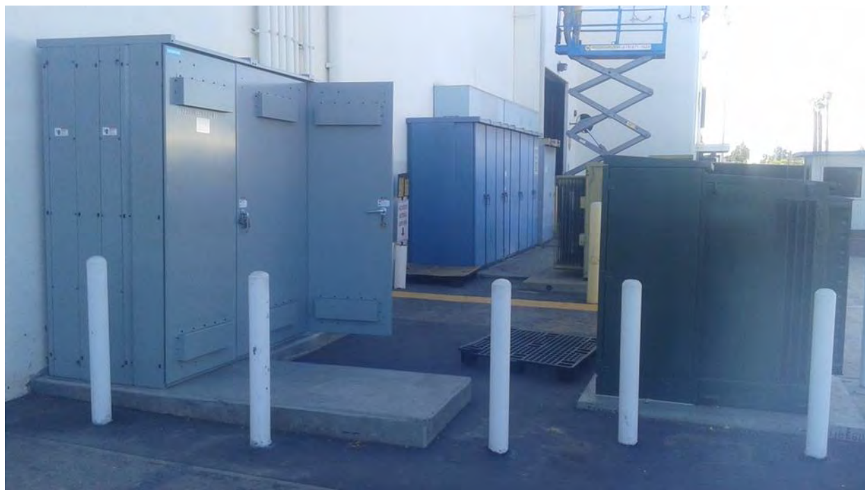
Figure 23. UPS San Diego EVSE supporting infrastructure
