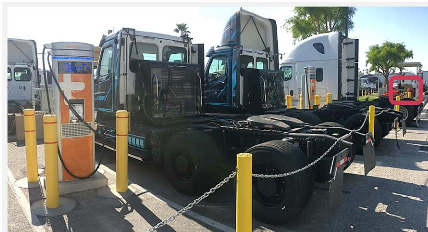
Figure 19. Heavy-Duty Vehicles and Chargers (Foreground) and Transformer (Background)
