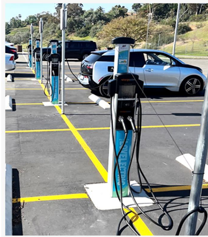
Figure 108. SDG&E Parks Pilot Los Palmas Park High Access Level 2 Charging
