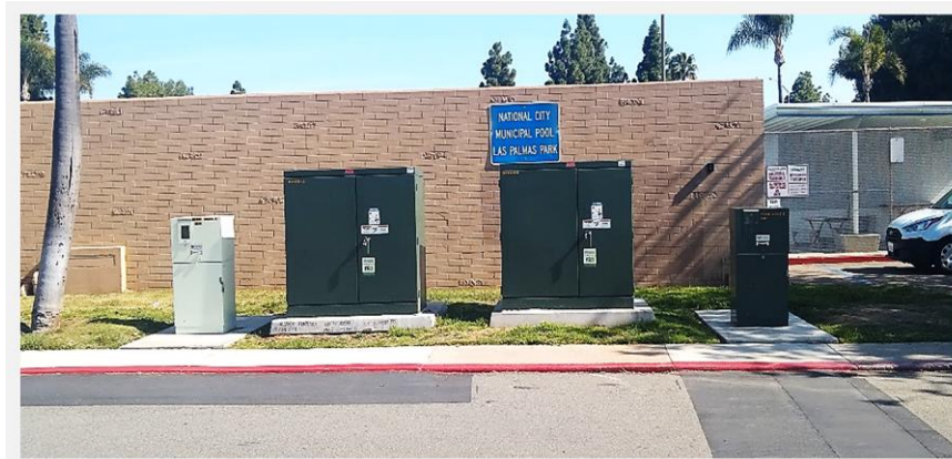
Figure 106. SDG&E Parks Pilot Site with Two Transformers and Two Meter Pedestals to Serve DCFC and L2 Charging
