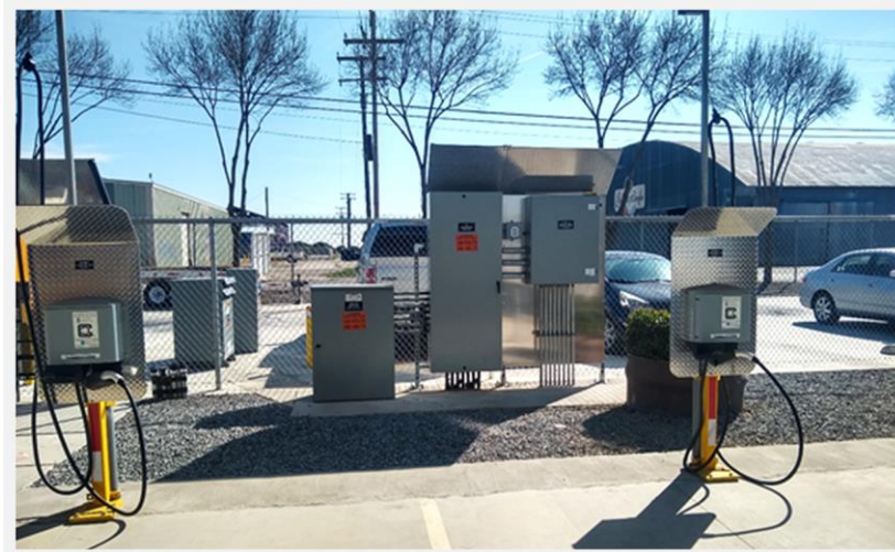
Figure 16. Charge Controller (and Switchgear in Background) to Enable Non-Networked EVSE
