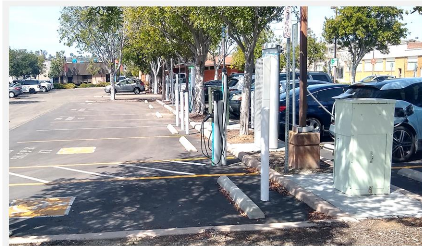
Figure 109. SDG&E Parks Pilot Site Example of ADA-Accessible Charger
