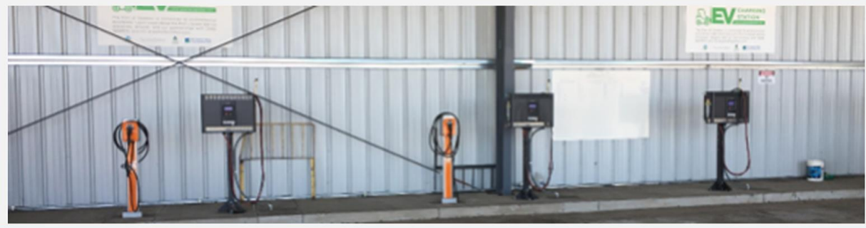
Figure 51. Forklift Charging Using a Mix of Legacy and New Equipment
