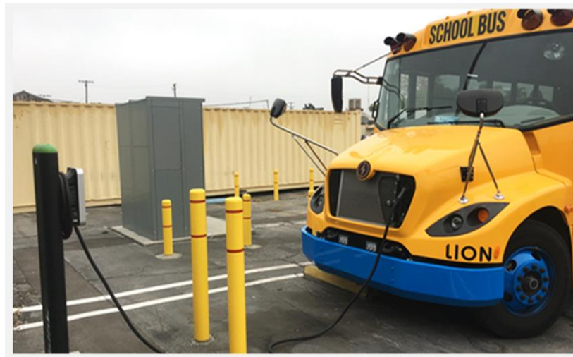
Figure 15. School Bus with Charger Station and Switchgear
