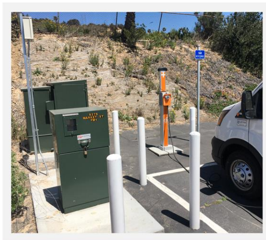
Figure 96. Electrical Switch Gear in Relation to EVSE
