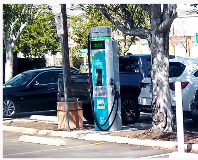
Figure 107. SDG&E Parks Pilot Site with Charging Stations Located to Reach Multiple Parking Spaces
