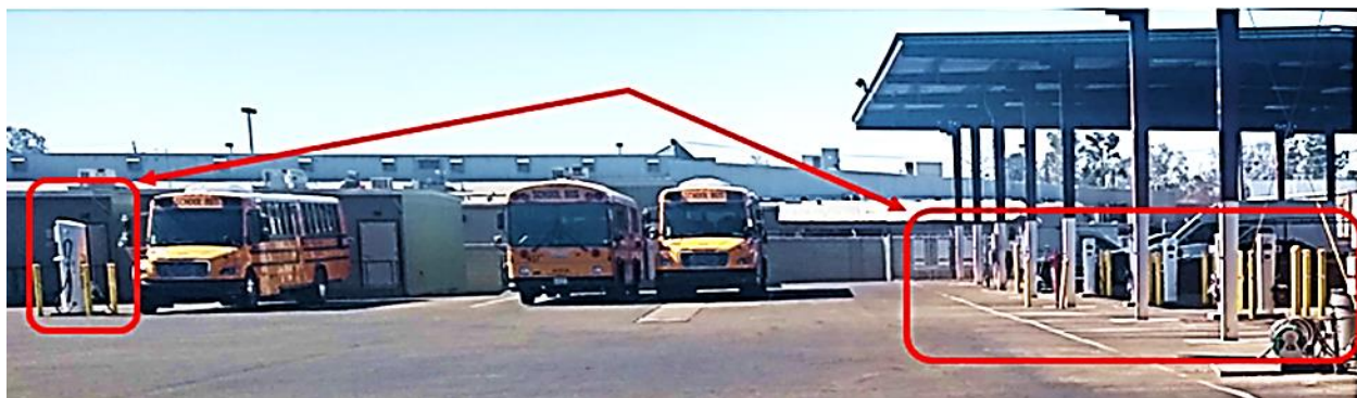
Figure 50. DCFC (left) and L2 (right) Charging with a Solar Canopy
