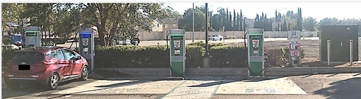
Figure 79. PG&E EV Fast Charge Program Public Charging Site in Tracy, California; Building Proximate
