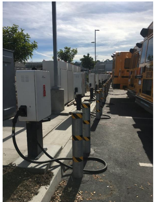
Site Layout Showing Nine of 12 Power Electronics Dispensers (small units) and Power Cabinets for 60 kW Rotational Charging (white boxes at image center)
