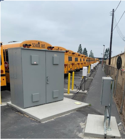
Switchgear, Nuvve Chargers, and Blue Bird RE Electric Buses
