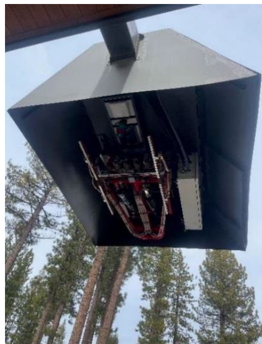
Figure 262. Liberty EV Bus Infrastructure Program Detailed View of Pantograph Mechanism and Protective Cover
