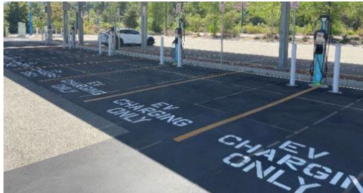
Figure 227. SDG&E Schools and Parks Pilots High-Access Location with L2 and DCFC Ports
