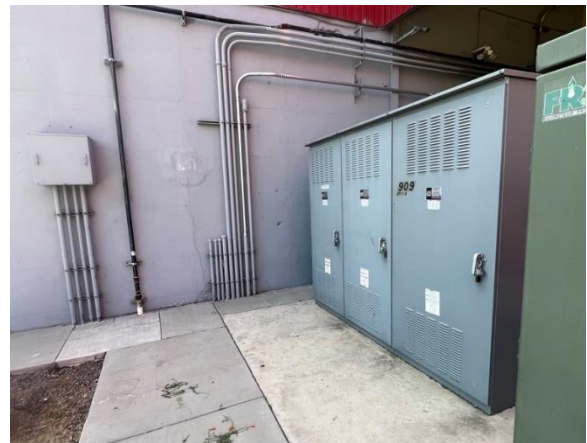
Switchgear and Conduit Run at Site 2
