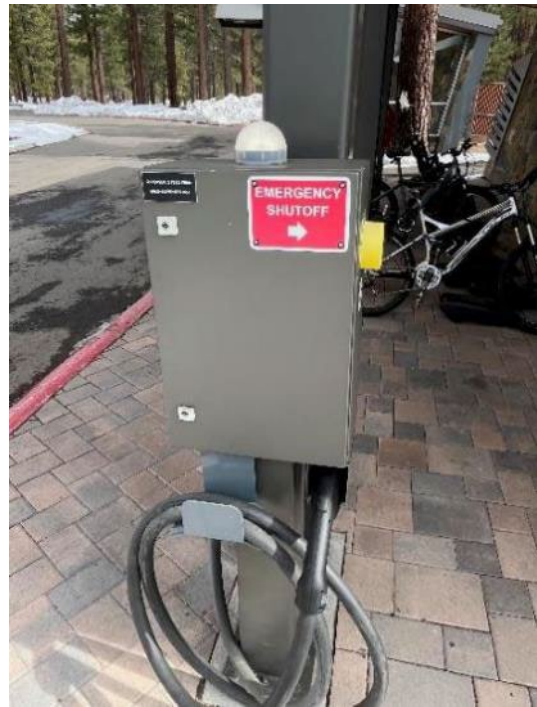
Figure 264. Liberty EV Bus Infrastructure Program CCS Dispenser at LTCC
