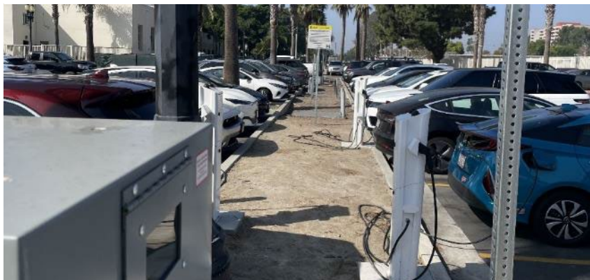
Figure 89. Example of High-Access Charging Layout
