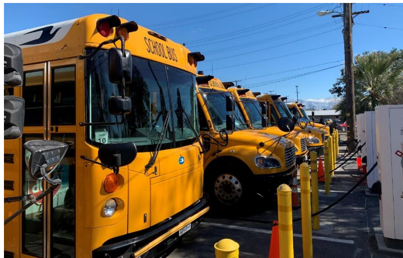
Site Layout Showing Four ABB Terra Units and Charging Thomas/Proterra Buses
