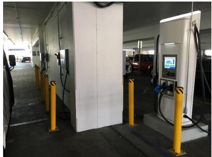
Site Layout Showing 2 Delta Electronic DC Wallboxes (left) and BTC Power DCFC (right)
