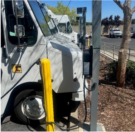
Class 6 Step Vans at Site 1, Showing Outdoor Parking Facilities and Pole-Mounted Chargers
