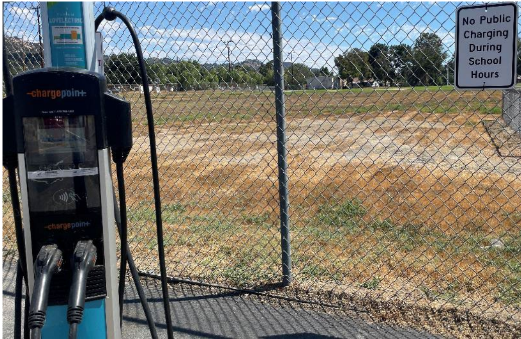
Figure 225. SDG&E Schools and Parks Pilots Example of School Limiting Use of Charging by Public
