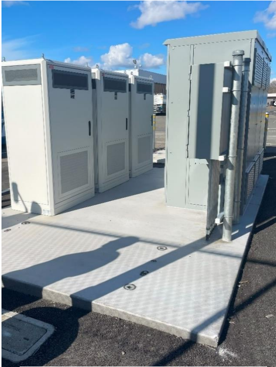
Three ABB 150 kW Chargers and Supporting Electrical Switchgear
