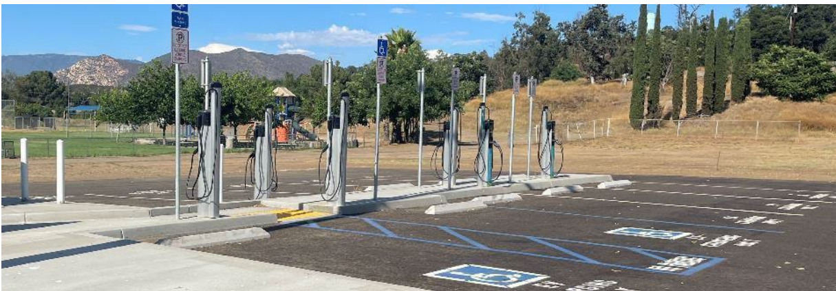
Figure 224. SDG&E Parks Pilot Rural - Tribal Charging Location
