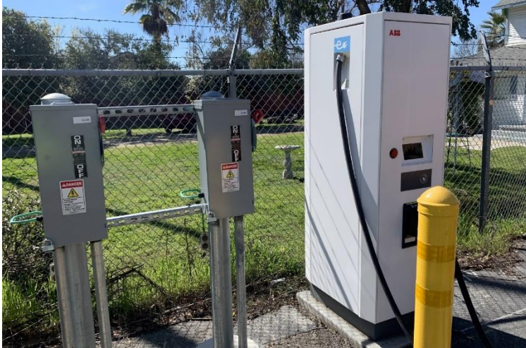
Standalone ABB Terra 50 kW Chargers and Associated Safety Shutoffs and Protective Bollard
