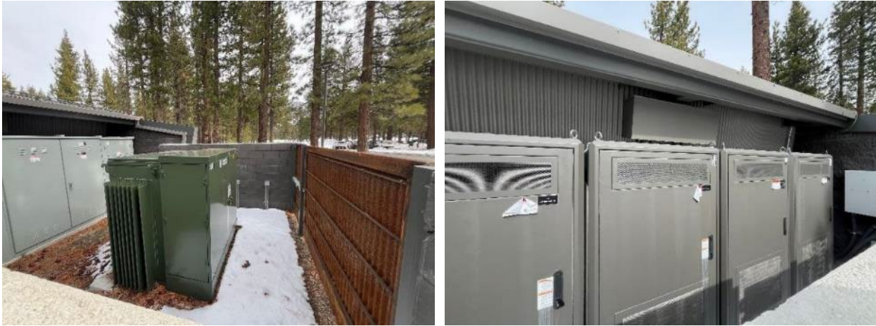
Figure 263. Liberty EV Bus Infrastructure Program Transformer and Switchgear (left) and DC Power Cabinets (right) for Electric Bus Charging at LTCC
