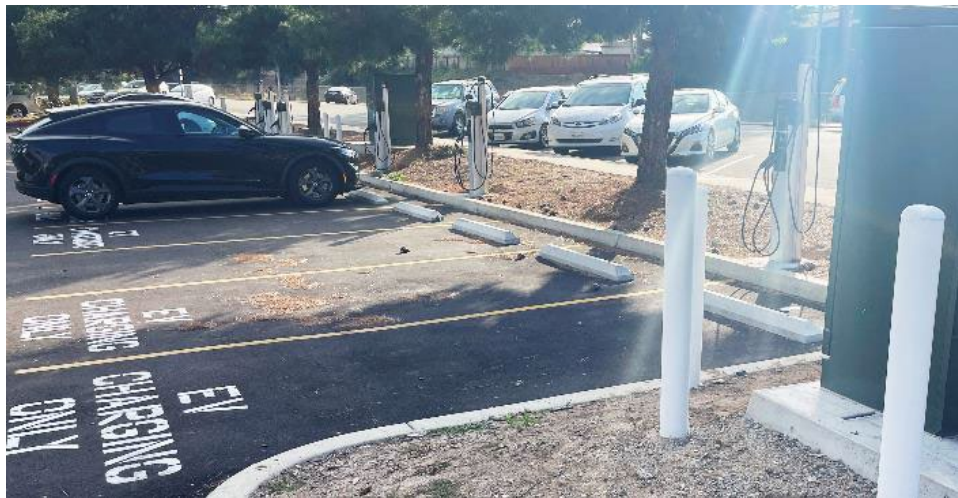
Figure 226. SDG&E Schools and Parks Pilots Example of High Access L2 Charging Layout
