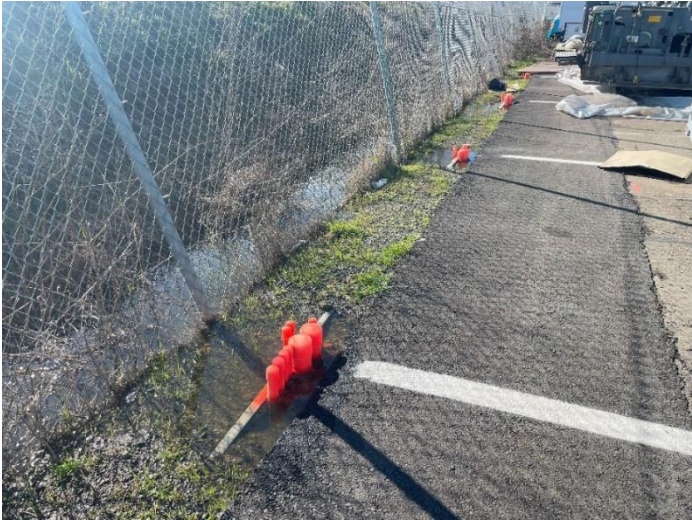
Charger Electrical Stub-outs (capped in orange) Showing Future Buildout Locations
