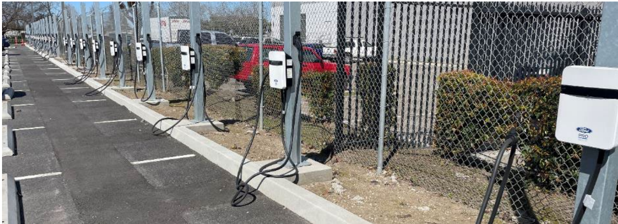
Figure 114. Large-Scale Deployment of Chargers at a Medium-Duty Site
