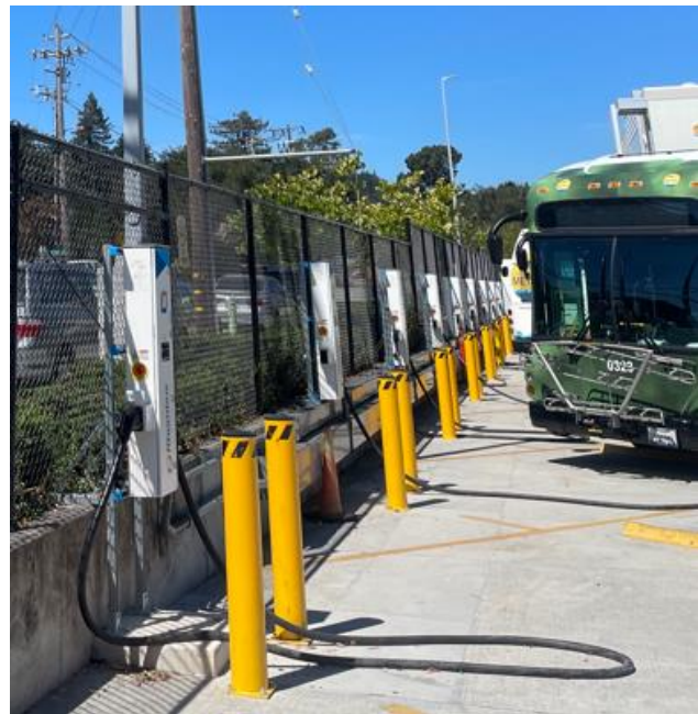
Figure 141. PG&E EV Fleet Program Transit Bus Charging Adjacent to Power
