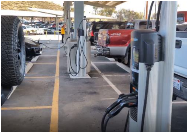
Figure 262. SDG&E Schools and Parks Pilots Example of High Access L2 Charging Layout
