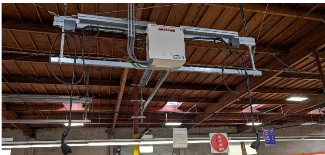
Figure 226. SDG&E PYDFF Program Site Overhead Low-Power DCFC Charger
