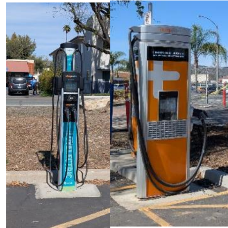
Figure 263. DCFC and L2 Chargers at an SDG&E Schools and Parks Pilot Site
