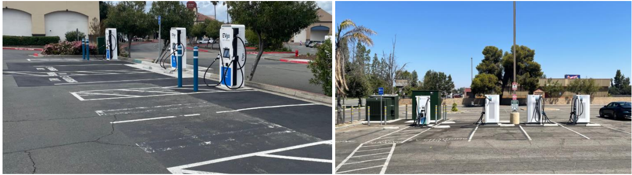
Figure 198. PG&E EV Fast Charge Program EY2024 Sites with Dual-Port EVSE (Left: 350 kW, Right: 180 kW)
