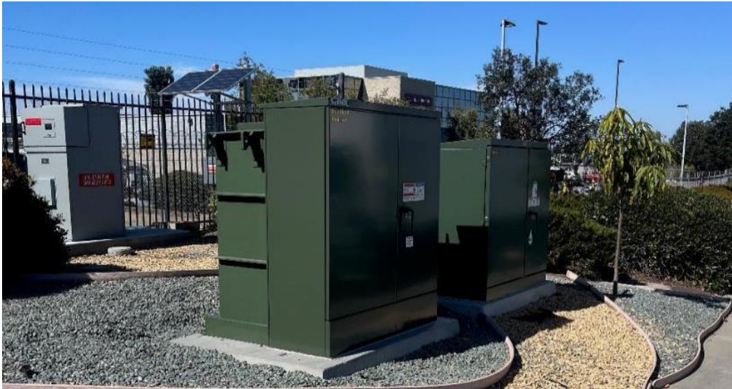
Figure 227. SDG&E PYDFP Program Site Transformer and Meter Pedestal
