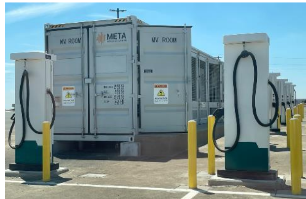
Figure 143. PG&E EV Fleet Program Containerized Power Solution and Several Chargers and Switchgear Pad and Island
