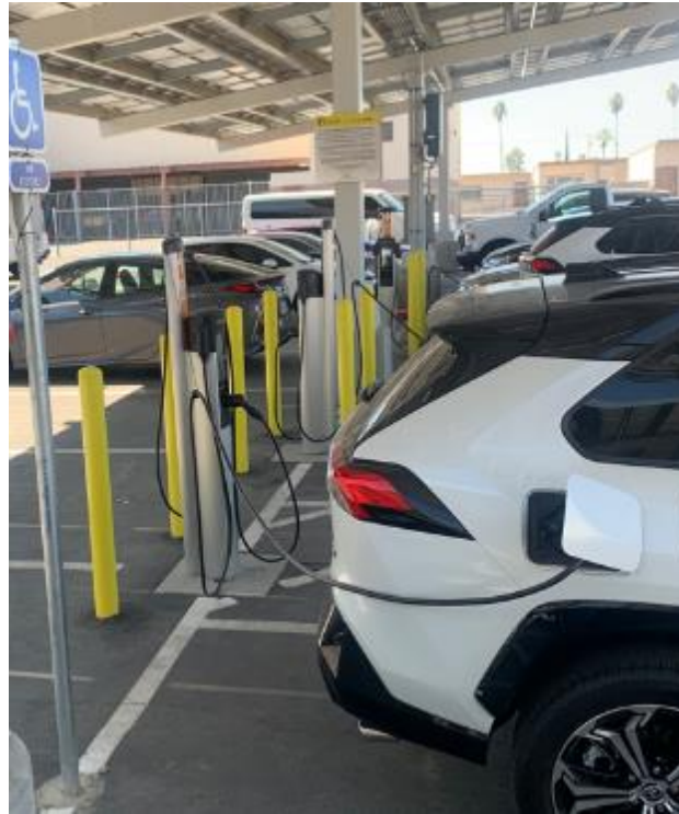
Figure 52. SCE Schools and Parks Pilot Head-to-Head Parking Resulting in Each Port Reaching 2.2 Spaces
