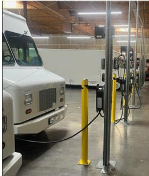
Figure 78. PG&E EV Fleet Program Indoor Parking at a Medium Duty Delivery Fleet Location
