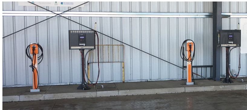
Charging installation at the site depot, showing 11-kW L2 chargers and 15-kW Xerator chargers
