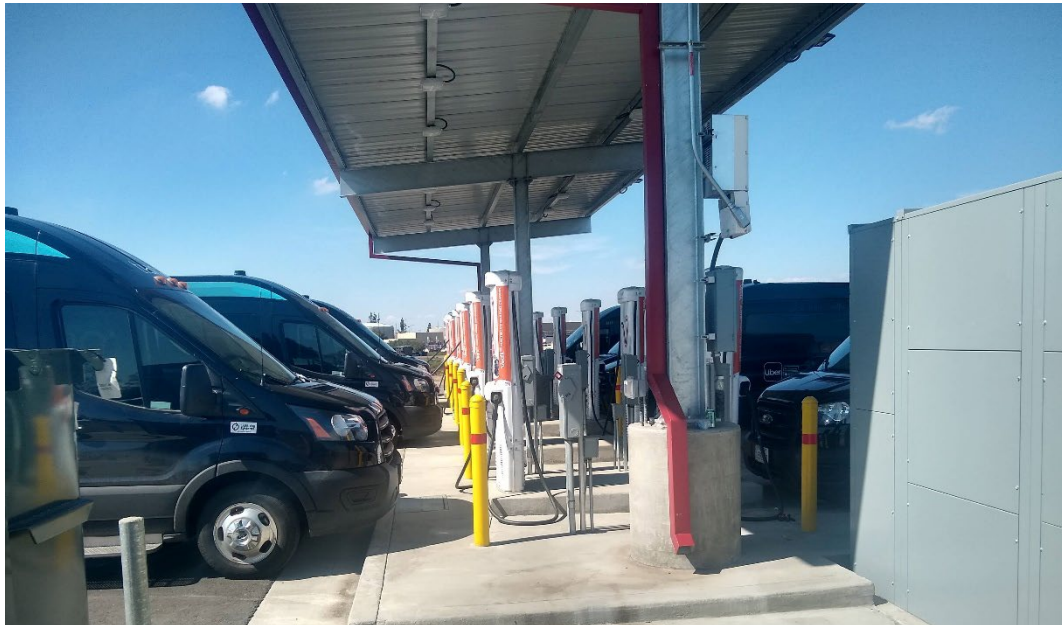
Charging installation at the site depot, showing chargers and multiple shuttle vans charging
