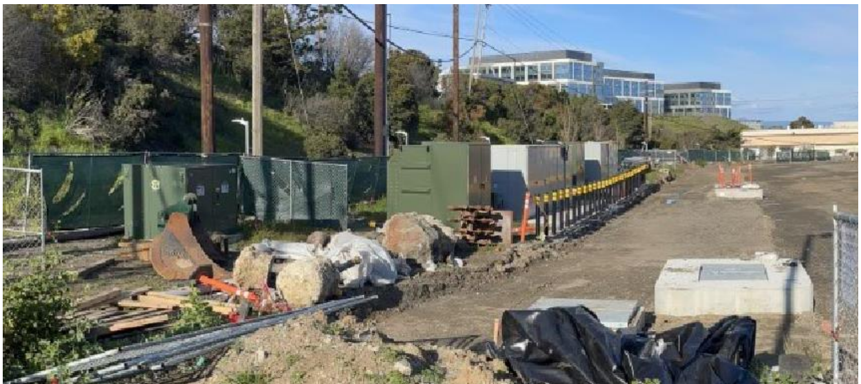
Figure 81. PG&E EV Fleet Program Inset of Above Photo Showing Transformers, Switch Gear, and Stub Outs
