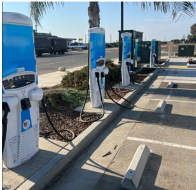
Figure 117. PG&E EV Fast Charge Program Charging Site Away from Building
