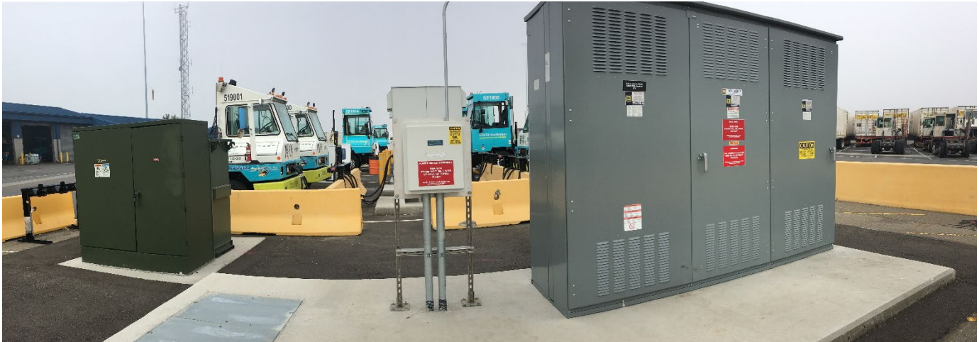
Charging installation at the site showing transformer (left), one three-port DCFC (center), switchgear (right), and several yard tractors (rear).
