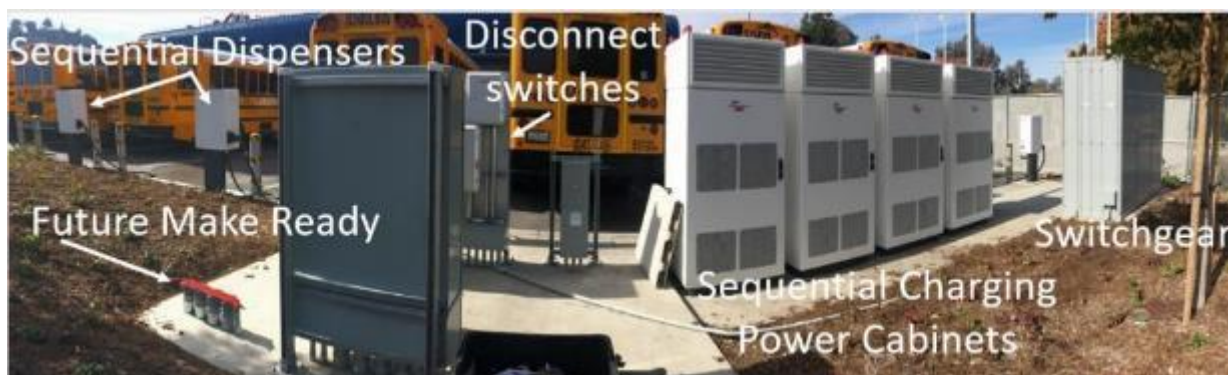
Figure 144. School Bus Site with Sequential Charging and Make Ready Infrastructure
