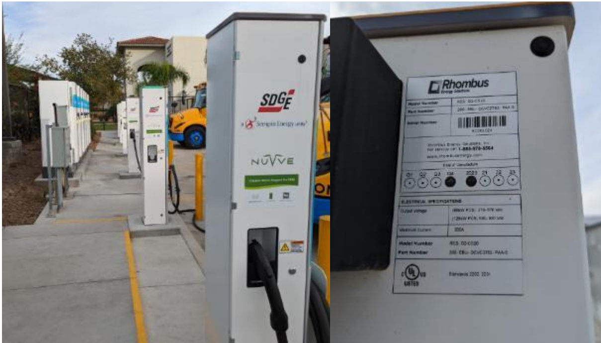
Figure 198. Nuve Rhombus DCFC Chargers (left: separate power cabinets and dispensers; right: Rhombus nameplate)
