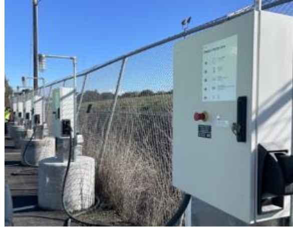
Figure 83. PG&E EV Fleet Program Sequential DCFC Dispensers
