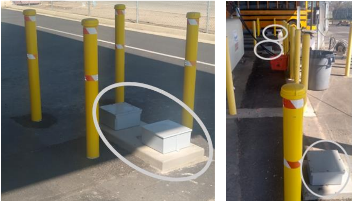
Figure 74. PG&E EV Fleet Program Preparation for Future Charging Stations
