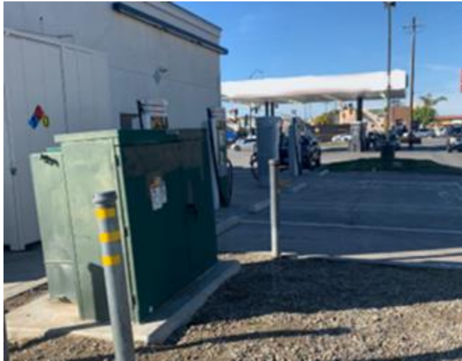
Figure 116. PG&E EV Fast Charge Program Charging Site Adjacent to Building
