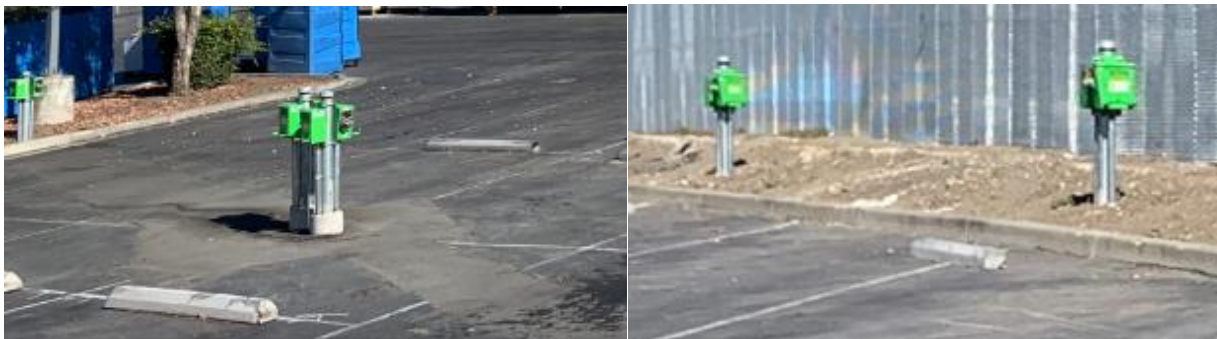
Figure 79. PG&E EV Fleet Program Example eTRU Ports
