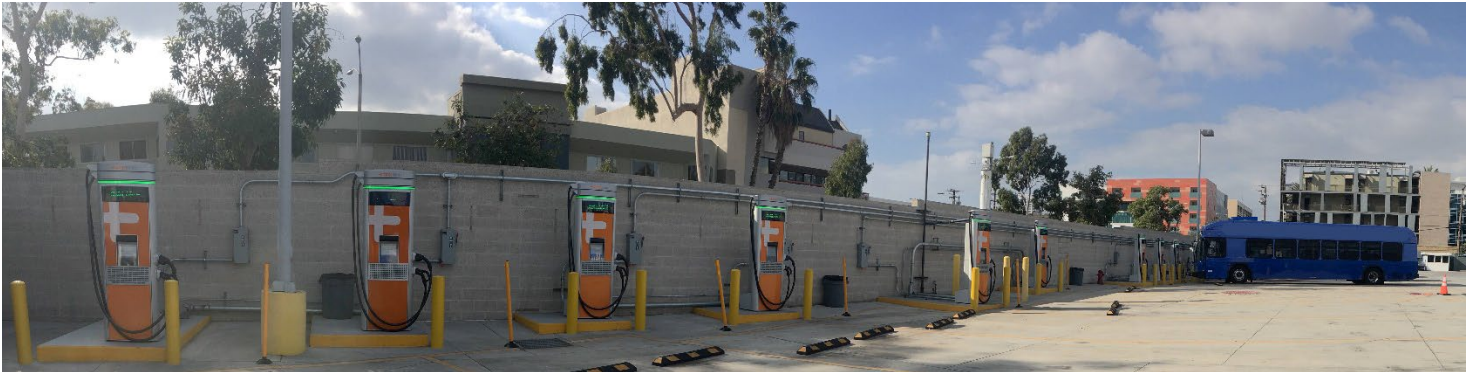
Charging installation showing chargers, above-ground conduit run, and a bus charging
