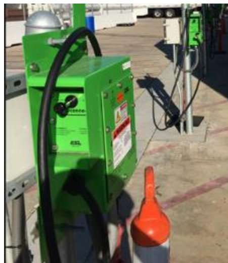
Figure 19. Electric Truck Refrigeration Unit Connector
