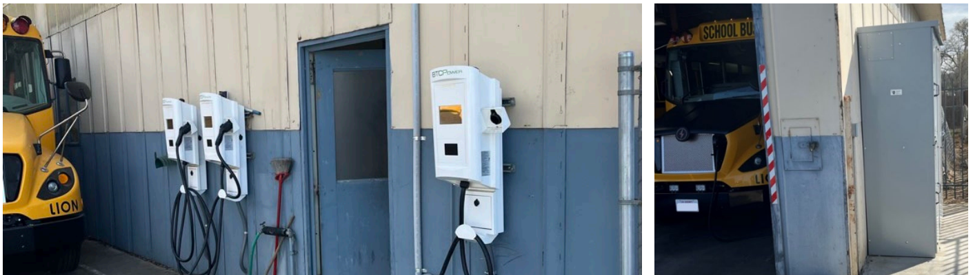
Charging installation at the site depot showing L2 chargers, above-ground conduit run, and switchgear
