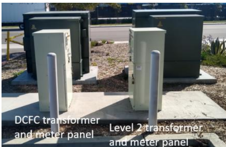
Figure 181. SDG&E Schools and Parks Pilots Site with Separate Meter Cabinets for Different Voltages for DCFC and L2 Chargers
