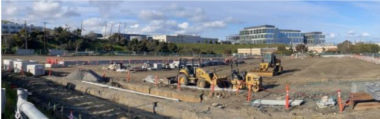
Figure 80. PG&E EV Fleet Program Large Site Doing Full Parking Lot Charging Infrastructure Build
