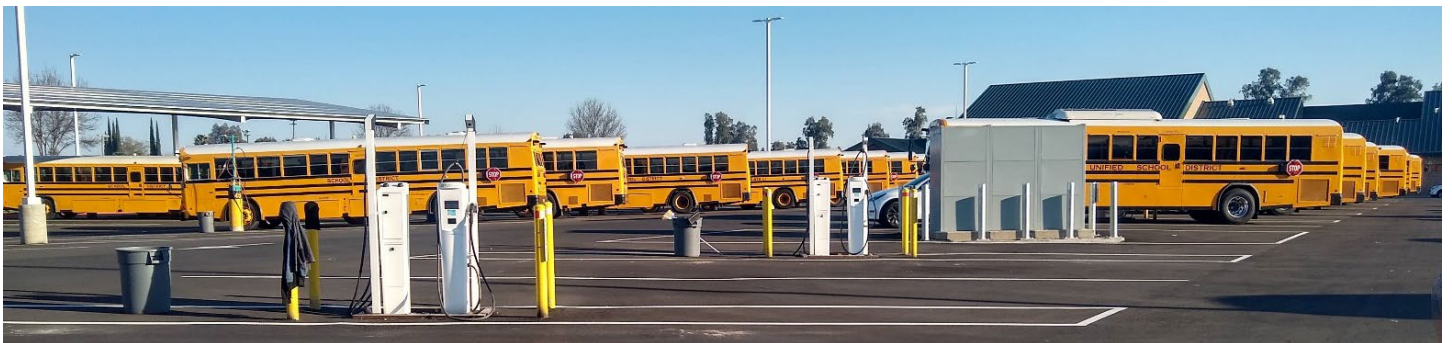
Charging installation at the site depot showing several buses, L2 charging stations (in white), and switchgear (in grey)
