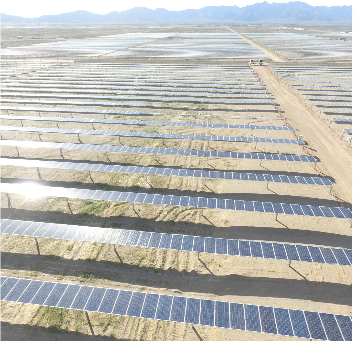
Photo Credit: NextEra Energy Resources
