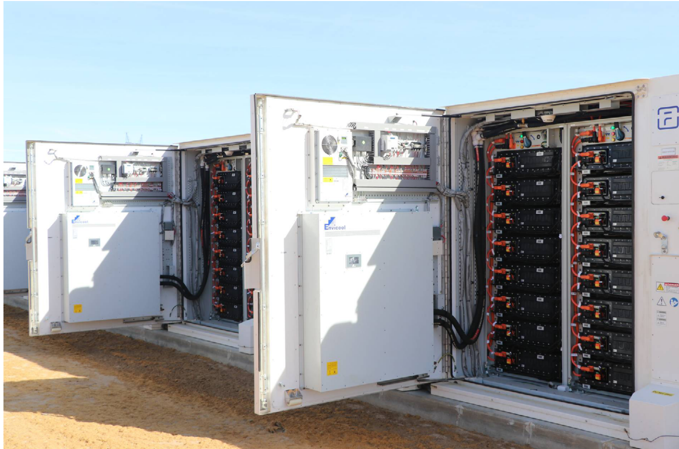
The 100 MW / 400 MWh Luna battery storage facility came online in August 2022 and provides enough energy to power roughly 75,000 Southern California homes for four hours every day.
