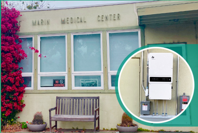
Above: Resiliency site West Marin Medical Center in Pt. Reyes with newly installed battery storage.
