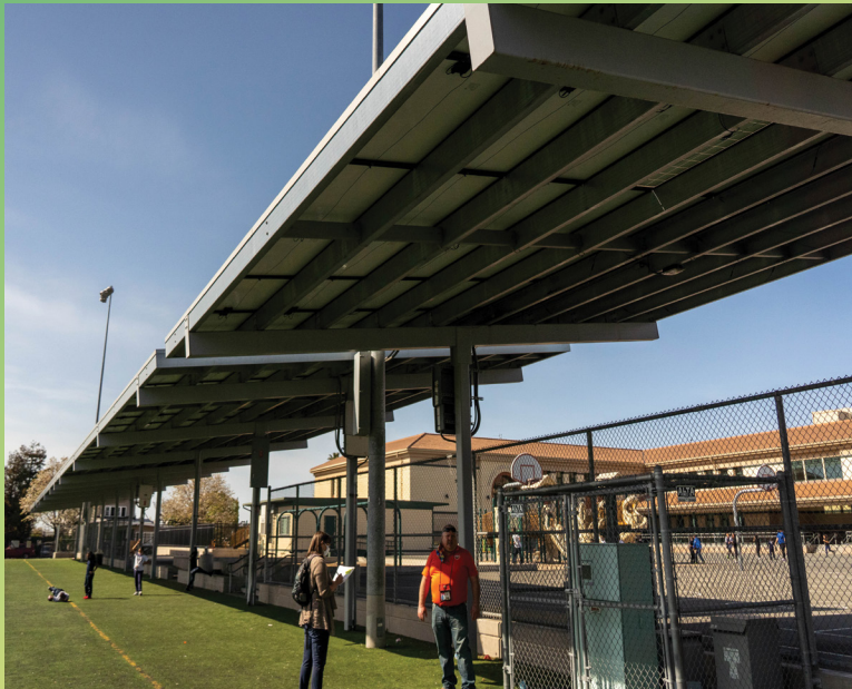
Below: Pittsburg Unified School District future battery storage site.
