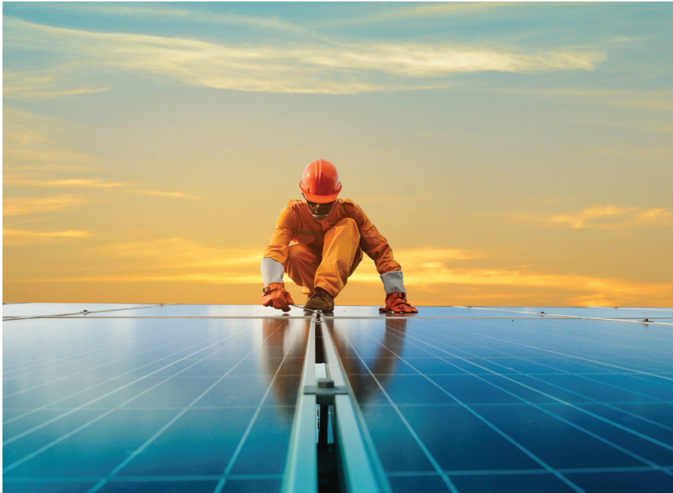
Desert Quartzite came online in December 2024, and is a 300 MW solar and 150 MW storage facility, serving as an essential component of CPA's energy supply. The facility will provide power for 145,000 homes in Los Angeles and Ventura counties.
