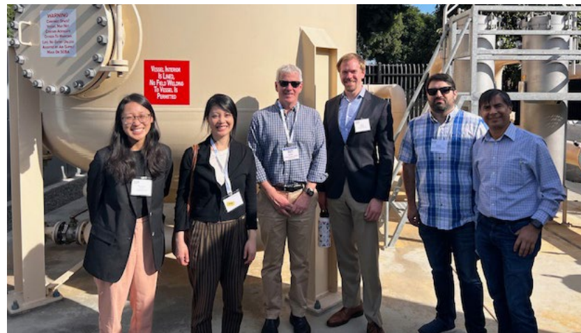
Commissioner Matthew Baker and CPUC staff tour a per- and polyfluoroalkyl substances treatment facility in Southern California on November 10, 2024.
