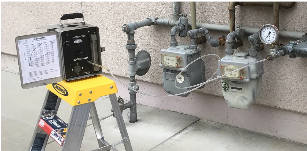
Natural gas meters connected to a testing device during a gas odorant intensity test.
