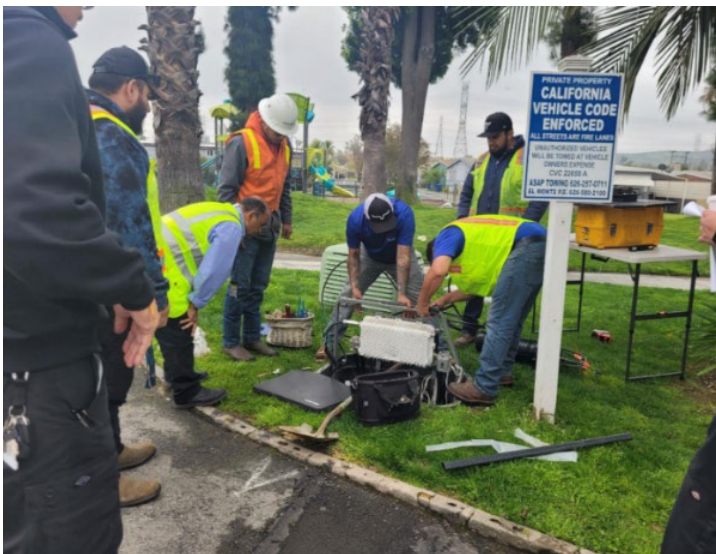
Figure 2: Charter Communications constructing last-mile fiber splices for the Brookside Mobile Home Park in Los Angeles County. Completed in 2023 and now has 190 broadband subscribers.
