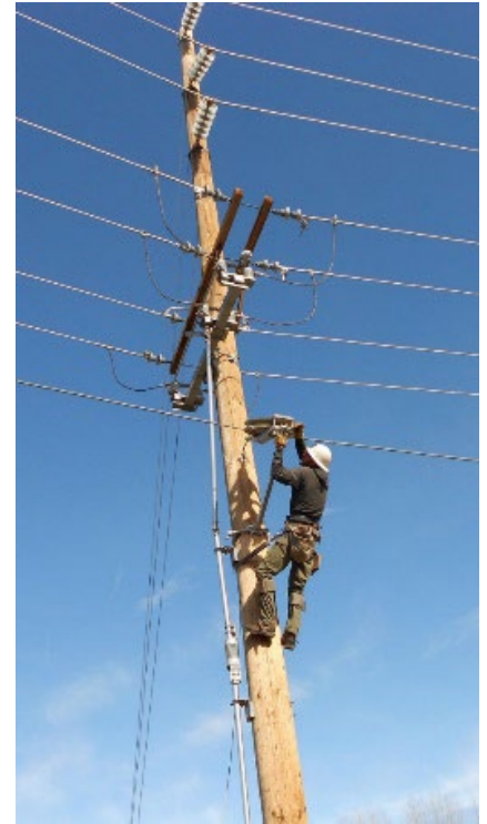
Figure 3: Hunter Communications placing fiber in Humboldt County for the Hoopa Valley Broadband Initiative Completed in July 2023 and currently active with 220 subscribers.
