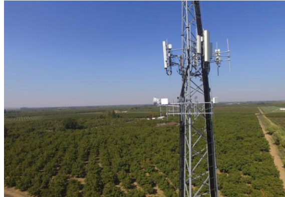
Figure 2: Last-mile tower constructed by Digital Path as part of the Placer and Sutter Counties project.
