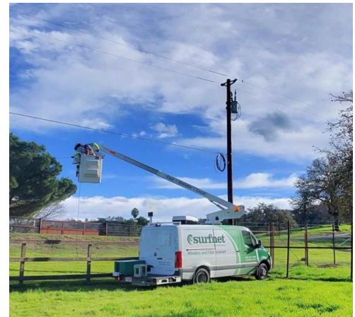
Figure 3: Surfnet Communications building new last mile infrastructure for their Three County Fiber project.
