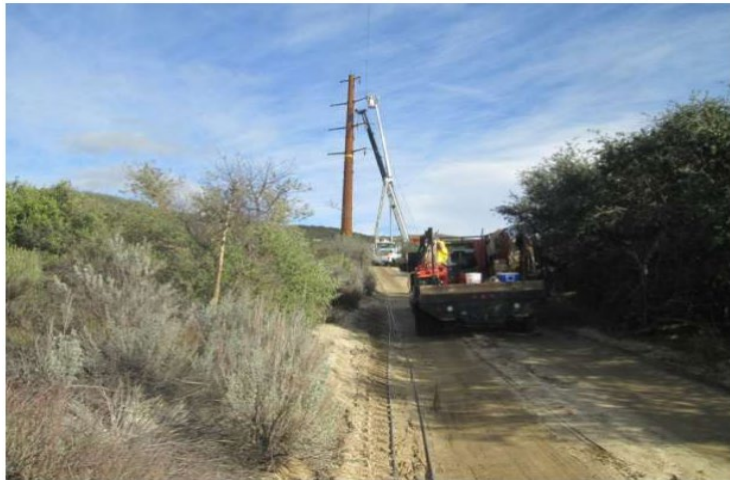
Typical power line (50-200 kilovolts)
