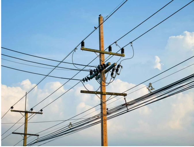
Typical distribution line ( <50 kilovolts [kV])
