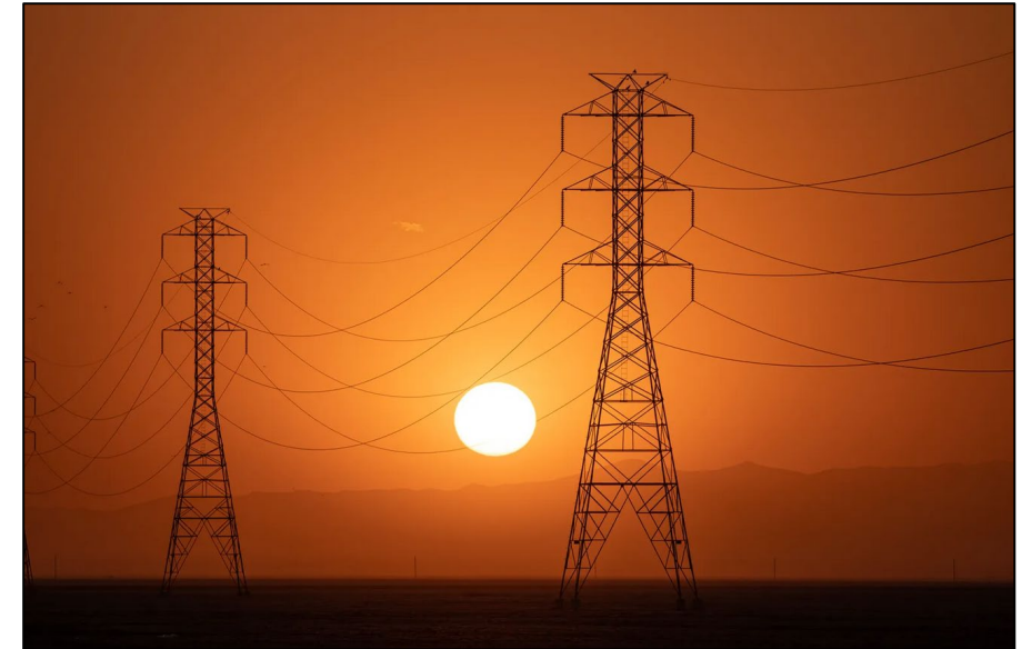
Typical transmission line ( >200 kilovolts)
