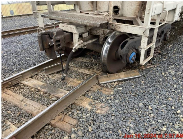
Broken rail where derailment occurred
