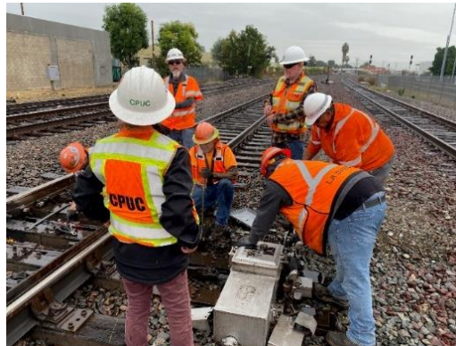
RSD inspectors observing operation of an electronically-controlled rail switch
