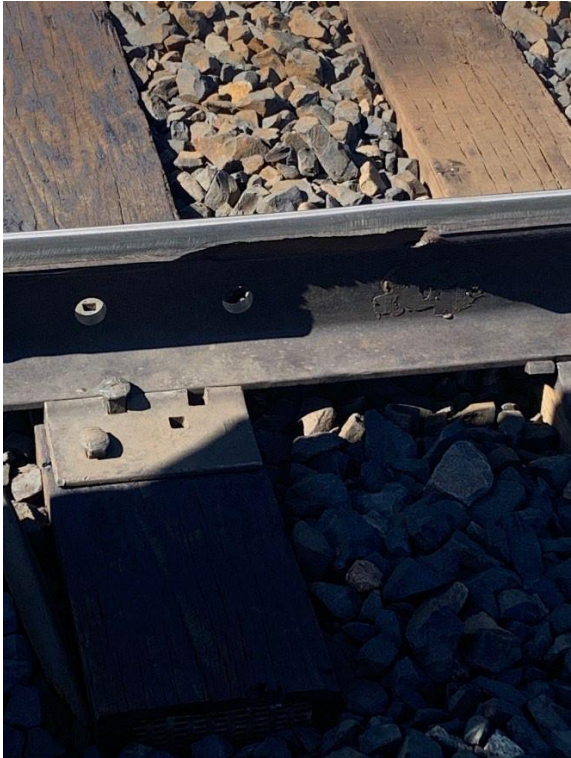
12-inch portion of broken rail
