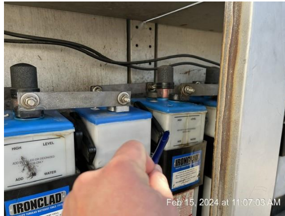
Defective battery cell in need of replacement
