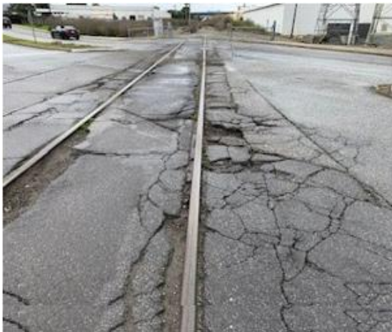
Damaged asphalt at crossing
