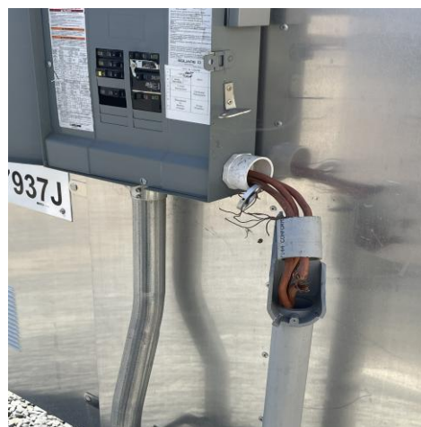
Vandalized wire housing exposing signal wires
