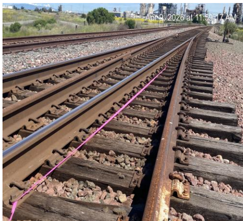
Before - Defective Fasteners
