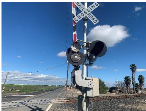
Crossing light hanging down
