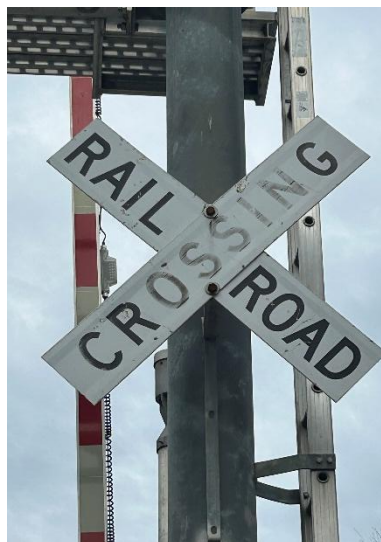
Faded crossbuck signage
