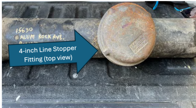
Figure 2. Post Incident photo – 4” Mueller Line Stopper with cap on (top view)
