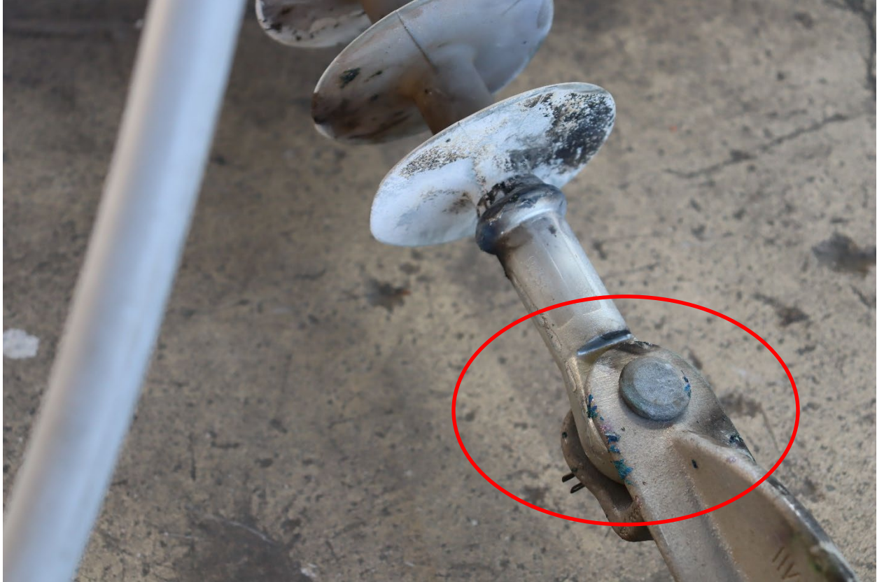
Figure 8. Mylar balloon marks on the B phase dead-end insulator/shoe assembly.
