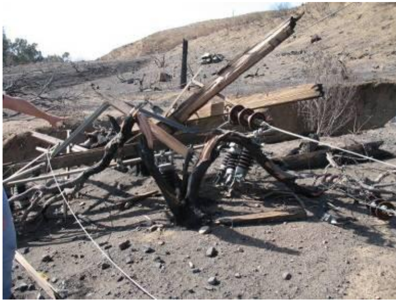
Photo 3 Damaged SCE Facilities
