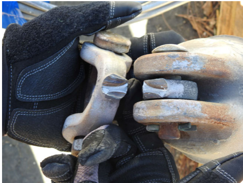
Figure 5: a photograph taken on October 25, 2019, at the evidence inspection at the SCE service yard, shows corrosion on the failed section of Y-clevis that supported the B-phase 220 kV conductor on tower M5-T2.
