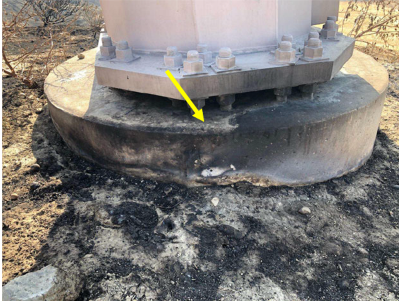
Figure 6: LAFD photograph showing evidence of unusual burning on one of the footings on Tower M2-T4.
