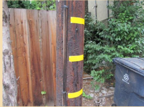
At this Location: Acceptable metal visibility strips attached 1 1/2" from ground.
