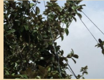
Guy overgrown by vegetation
