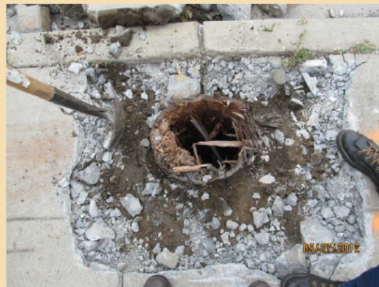
After extraction showing below ground deterioration
