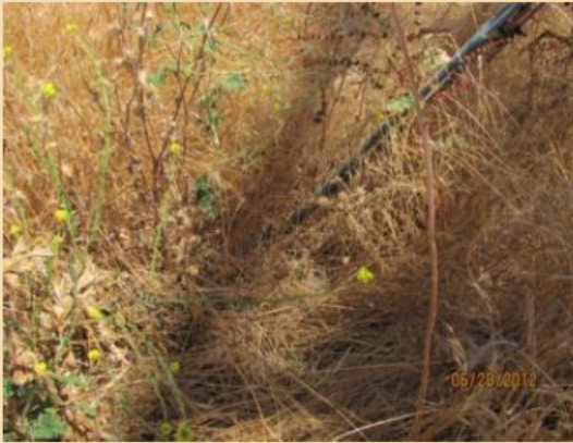
Before: Vegetation covers anchor
