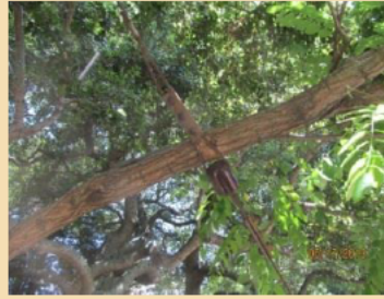
Guy grounded by vegetation
