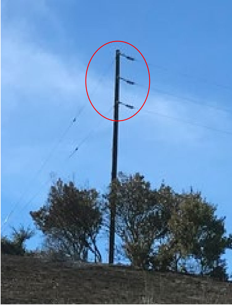
Figure 5: Pole No. X10282E with conductors in a vertical configuration, circled in red (Source: SCE).
