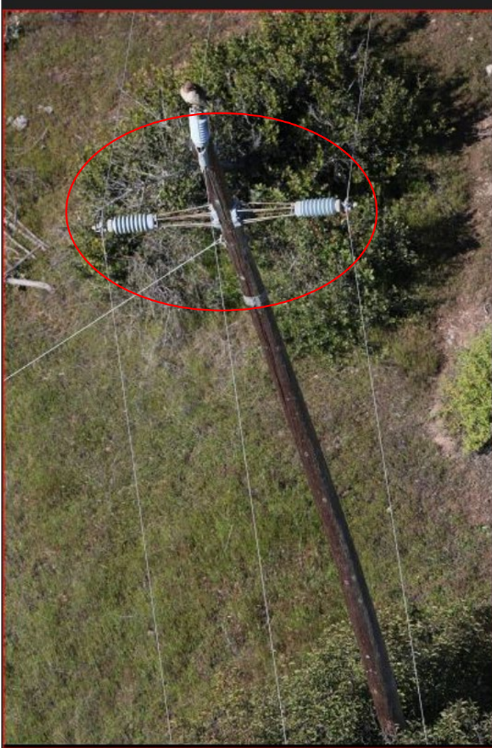
Figure 6: Pole No. X10703E with conductors in a horizontal configuration, circled in red (Source: SCE).
