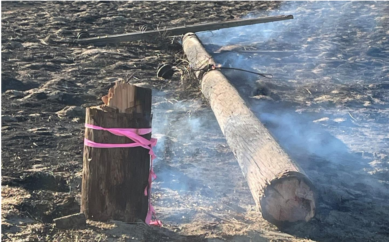
Figure 3: Pole No. 1714303E downed at Incident Location on November 9, 2023.
