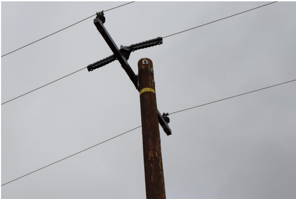
Figure 4: Replaced Pole No. 1714303E and equipment as seen by SED on November 16, 2023.
