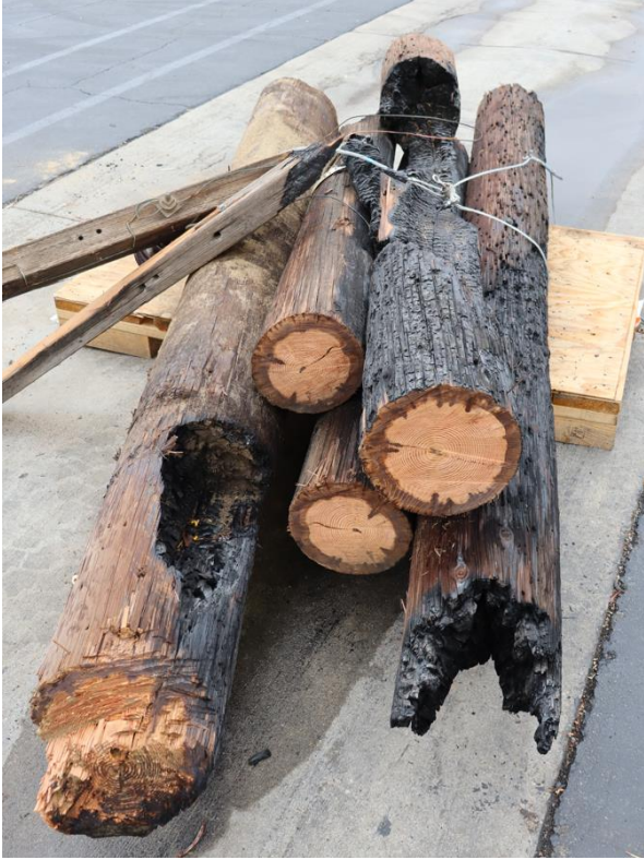
Figure 6: Pole No. 1714303E cut into sections for transportation and stored at the SCE yard.
