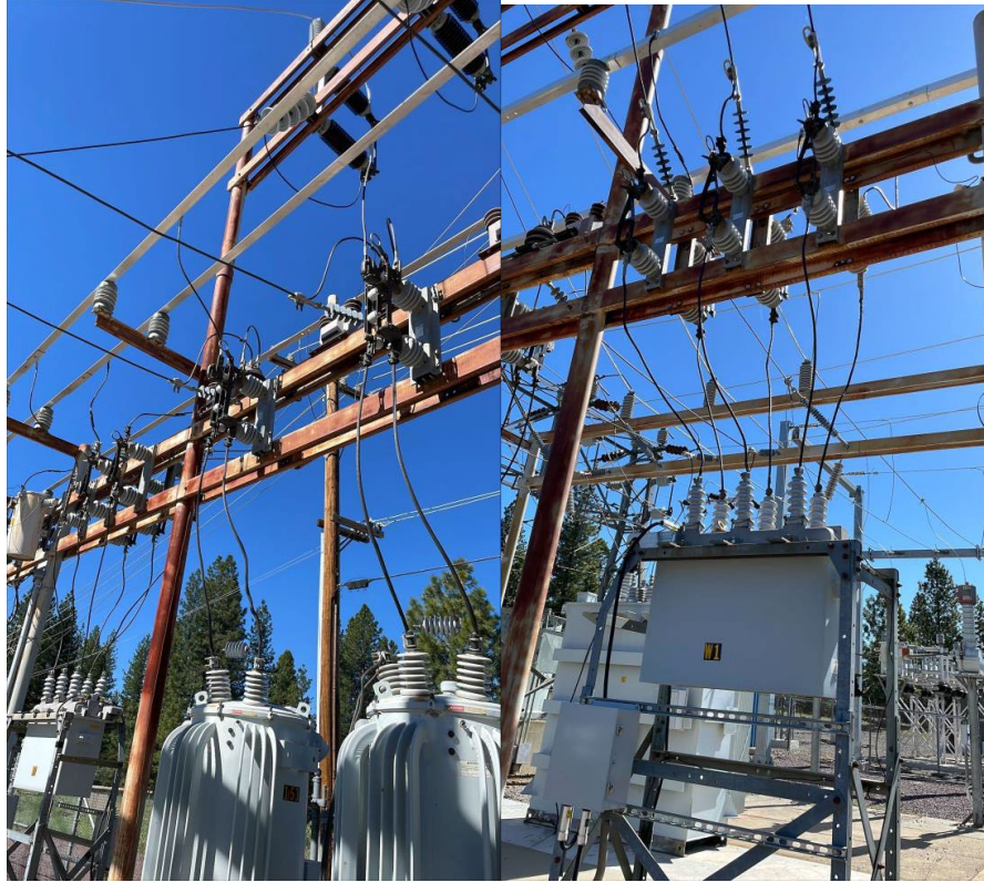
1.2. There are idle conduits on the ground that are damaged and have exposed wiring.
