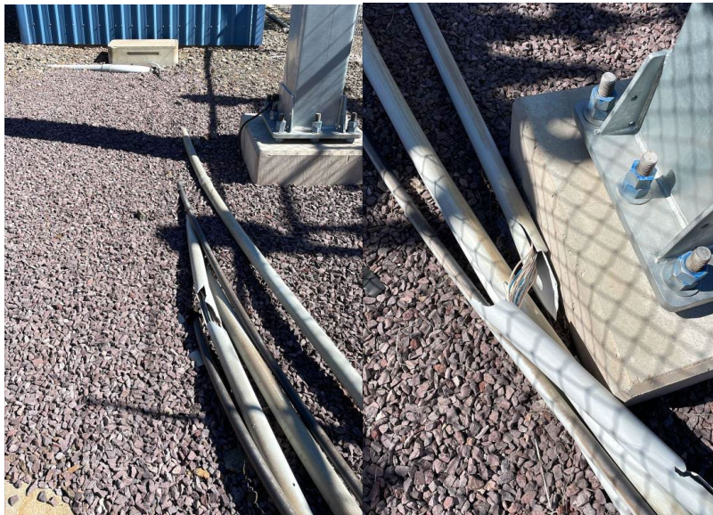
1.3. Modulation transformer is missing a high voltage sign.
