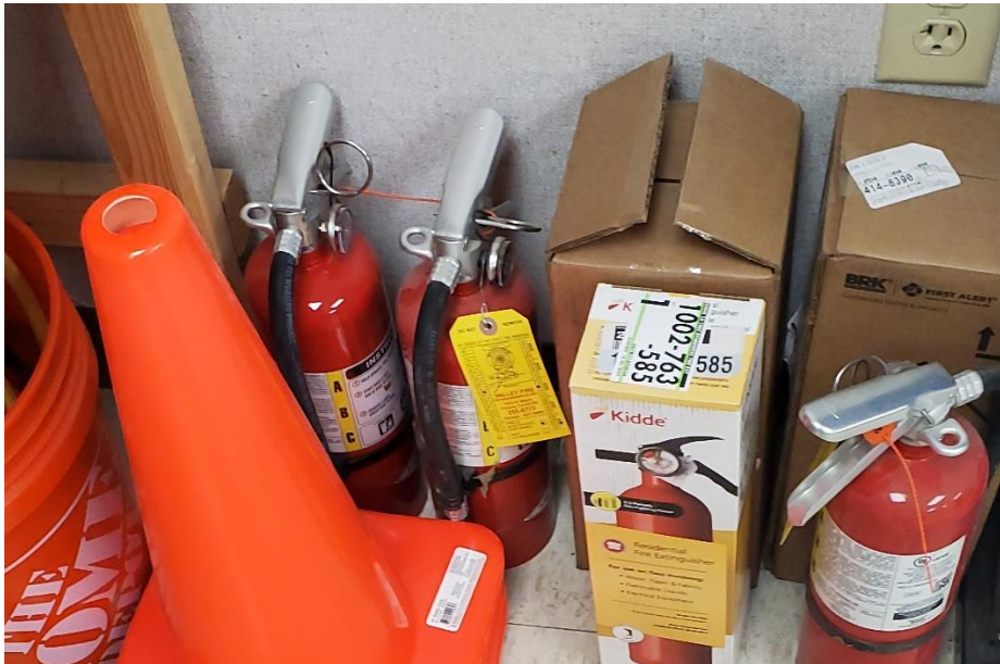
Figure 5: Spare fire extinguishers not being inspected.
