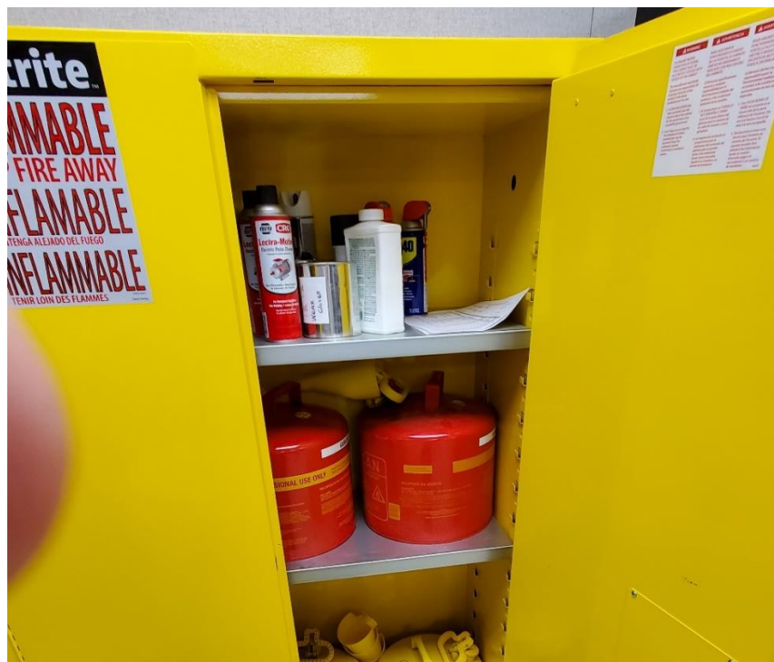
Figure 4: No self-closing on the Flammable Material Cabinet.
