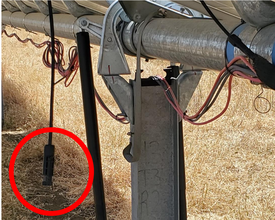
Figure 7: Broken connector hanging off solar panel.
