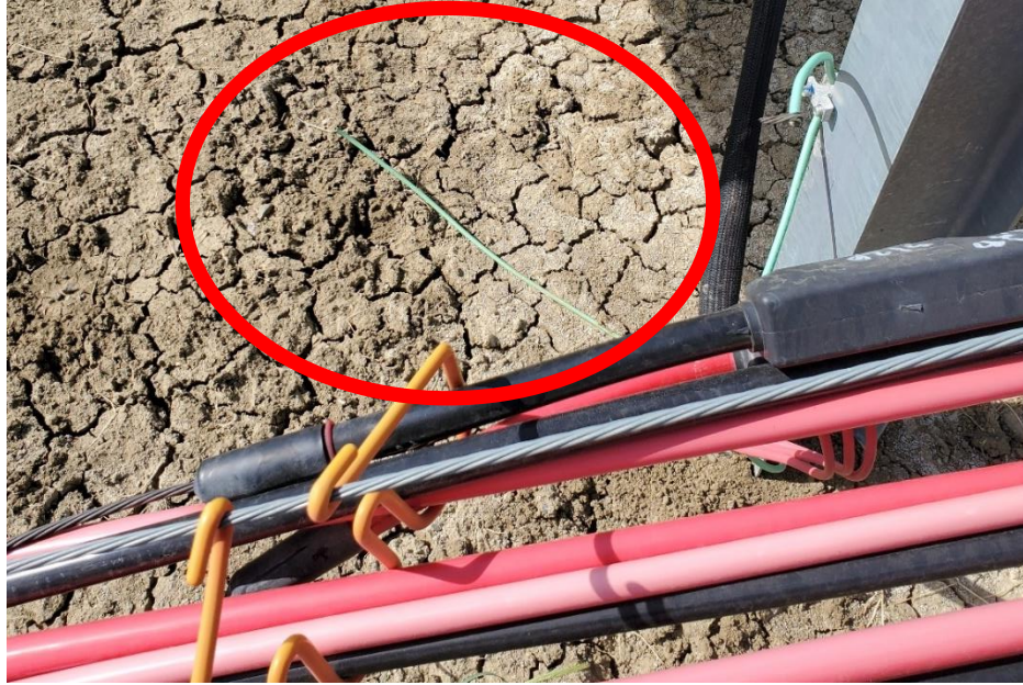
Figure 8: Example of broken ground observed throughout the Plant.
