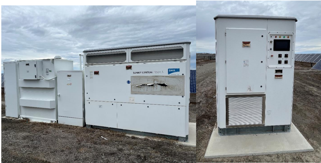
Figure 2: Inverter with deteriorated/faded high voltage signage at Array 2.
