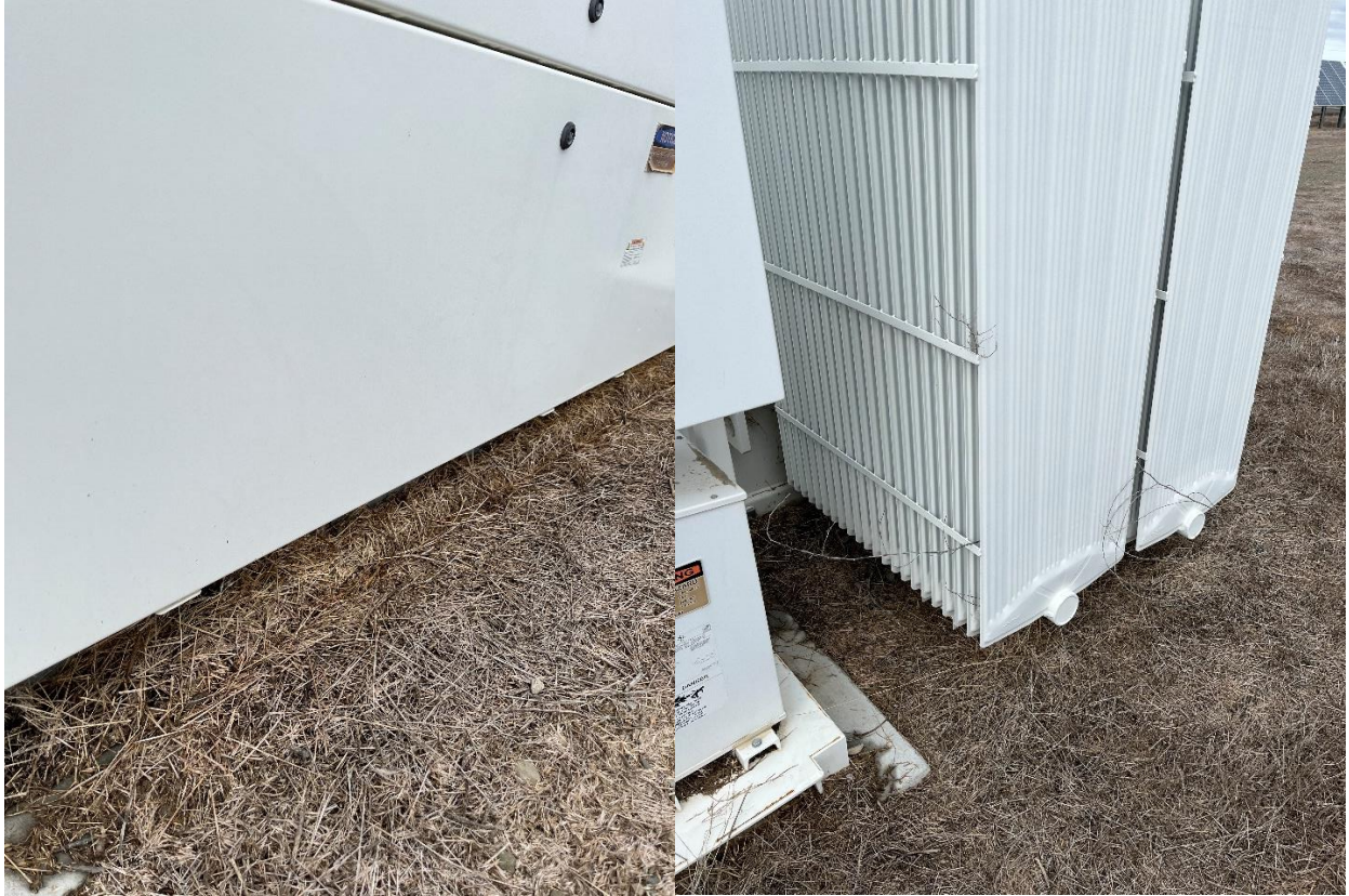
Figure 6: Overgrown vegetation at Inverter
