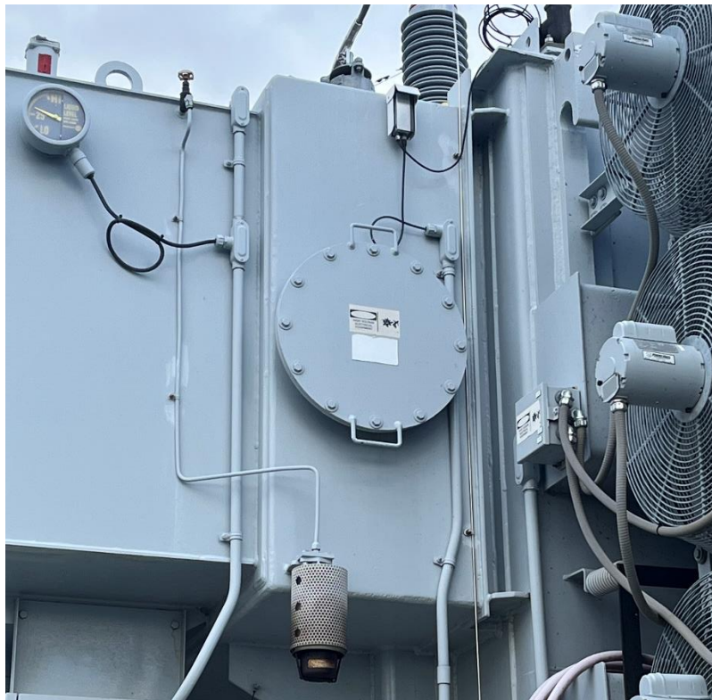
Figure 4: Confined space sign on manhole in substation is deteriorated/faded.
