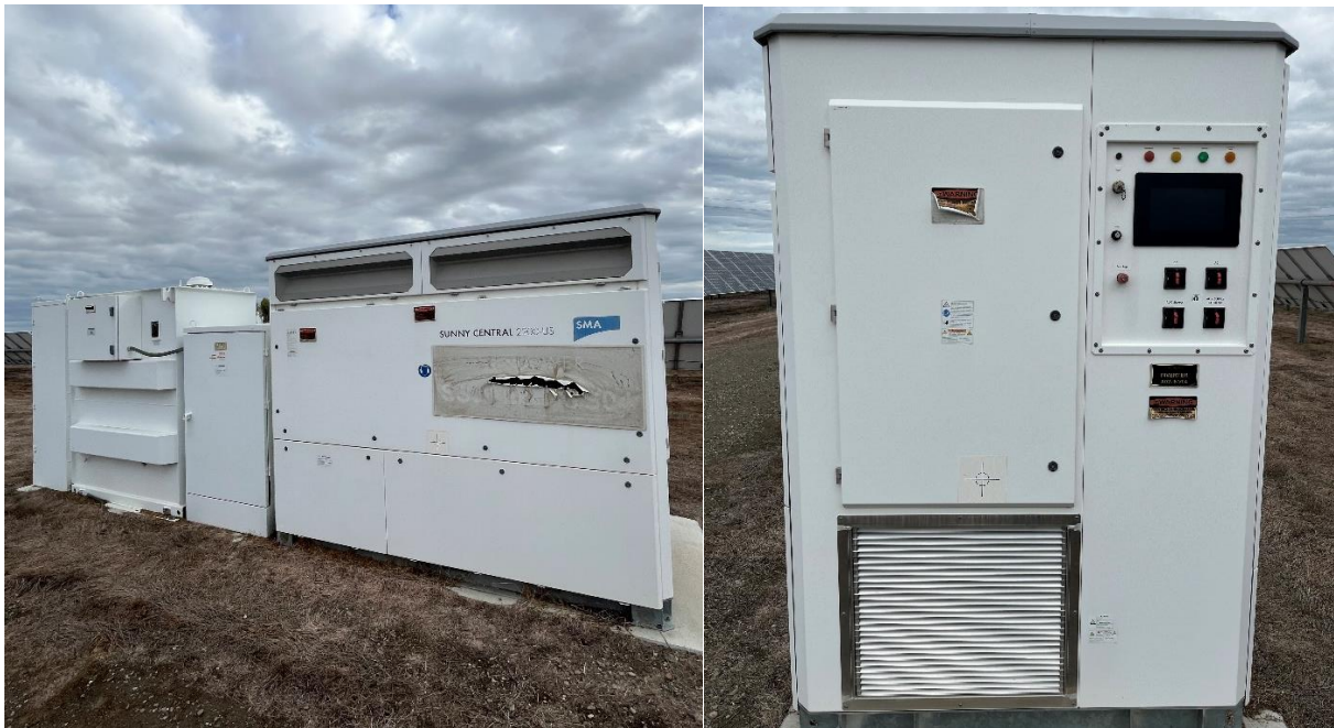
Figure 3: Inverter with deteriorated/faded high voltage signage at Array 3.
