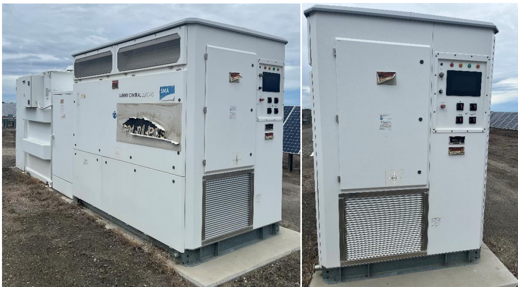
Figure 1: Inverter with deteriorated/faded high voltage signage at Array 1.
