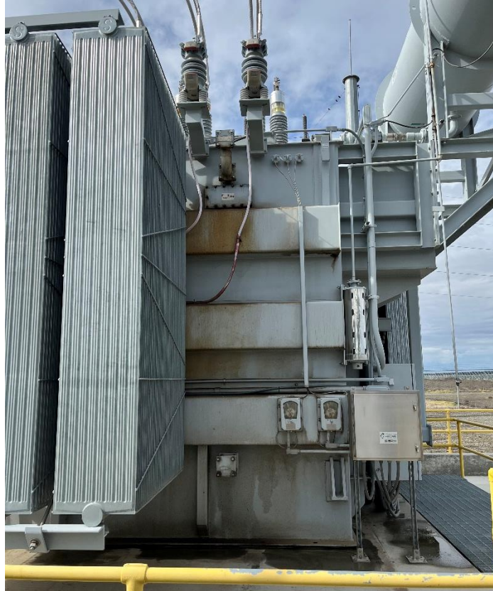
Figure 5: Oil leak at the low side flange of the main transformer.
