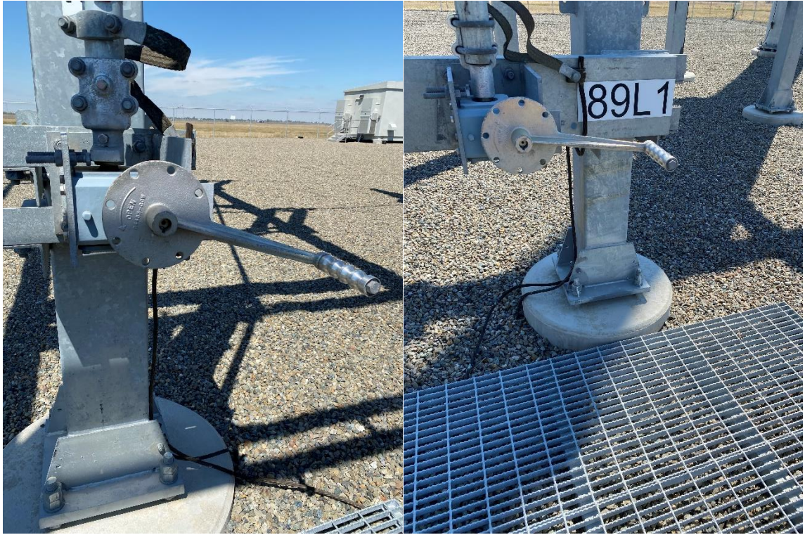
Figure 7: Two examples of unlocked disconnect switch cranks.
