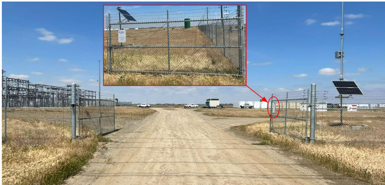
Figure 11: The current emergency contact sign is difficult to see upon entry.
