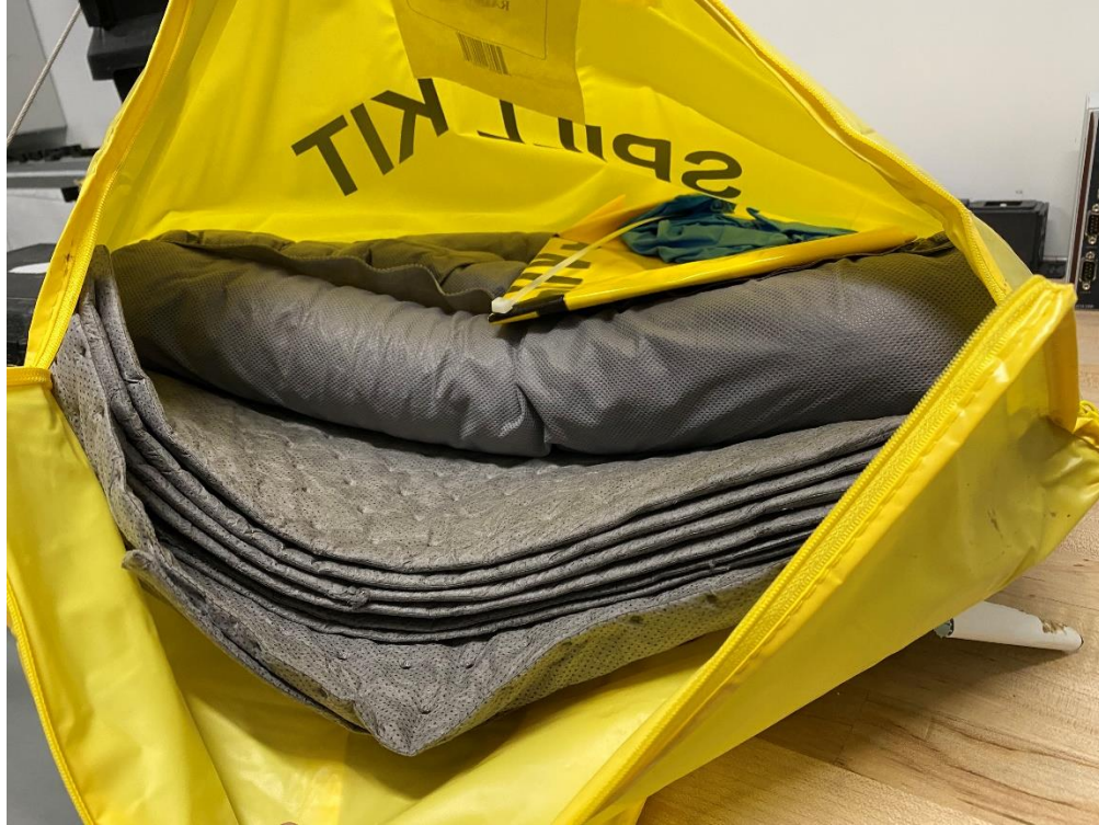
Figure 9: The spill kit in the substation control room is missing goggles.
