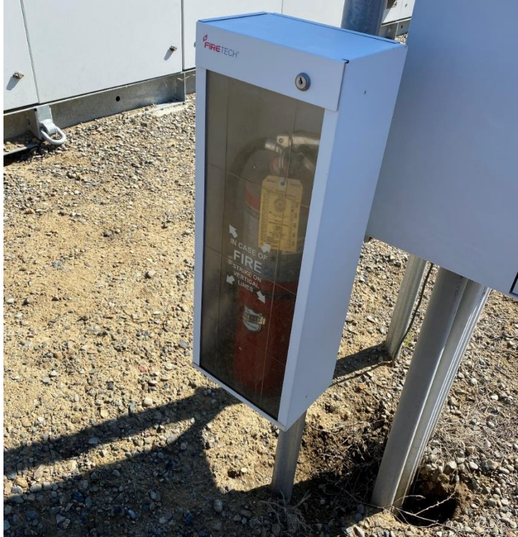
Figure 2: The fire extinguisher enclosure near one of the BESS inverters lacks a way to safely break the glass open.
