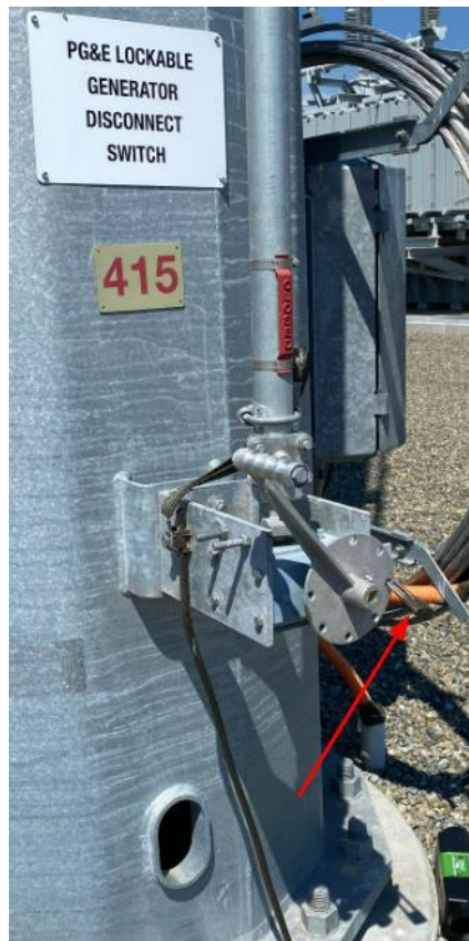
Figure 8: PG&E's disconnect switch is locked in the same substation yard.
