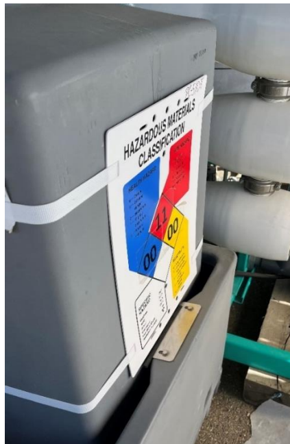
Figure 31: The PermaClean tank has an erroneous NFPA hazard diamond.
