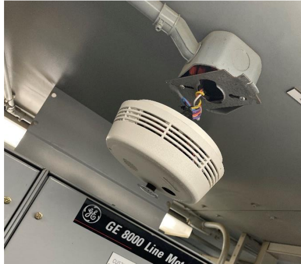
Figure 11: Loose smoke detector in the MCC.
