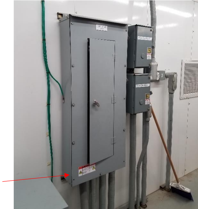
Figure 1: Electrical hazard 110/206 V breaker box door was open in the Unit 1 MCC.
