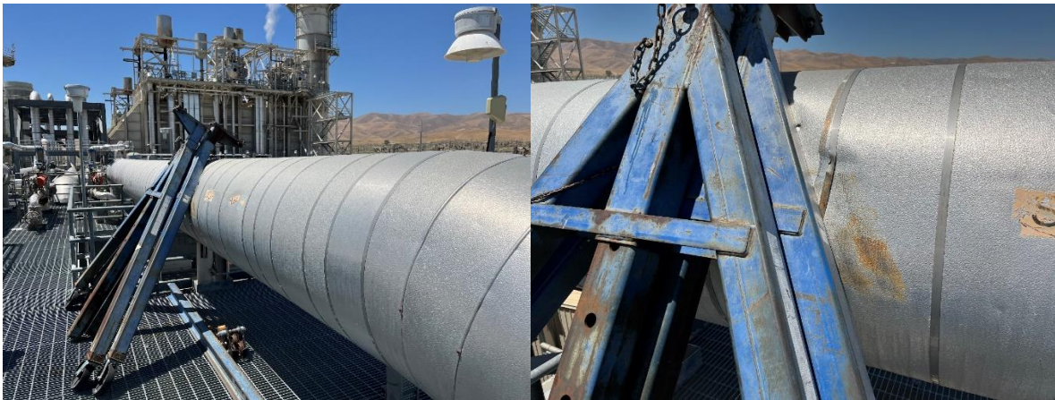
Figure 25: Equipment not in use stored against insulated pipes
