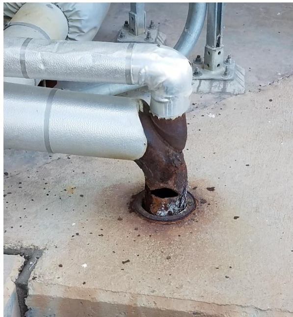
Figure 17: Flash drain for the evaporator cooler at Unit 1 and 2 has a hole due to corrosion.
