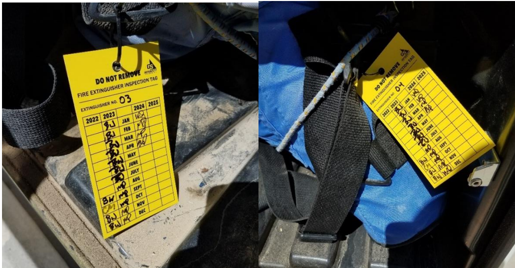
Figure 9: Two escape respirators are missing May 2024 monthly inspections.
