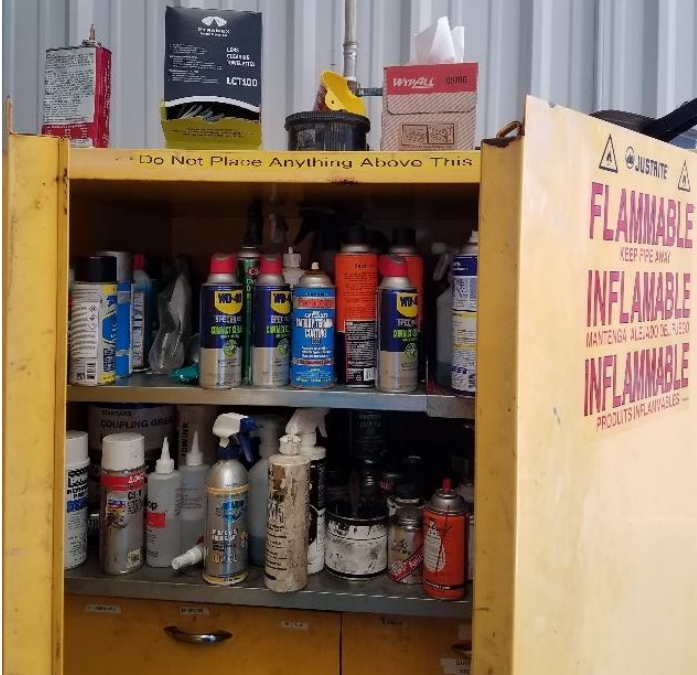
Figure 12: Machine shop flammable material cabinet has items stored on top.
