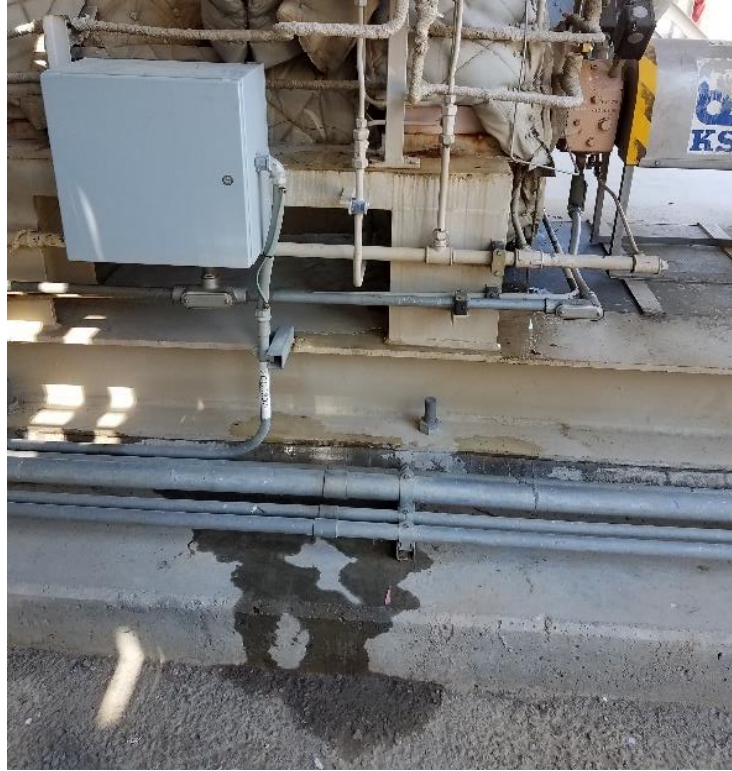
Figure 20: Boiler feed pump 201B has a water leak.
