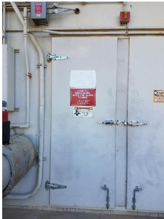
Figure 30: The Unit 1 STG has a faded/deteriorated danger sign and hearing protection sign.
