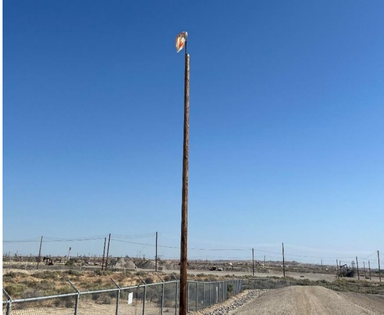
Figure 10: Damaged/deteriorated windsock on the west side of the property.
