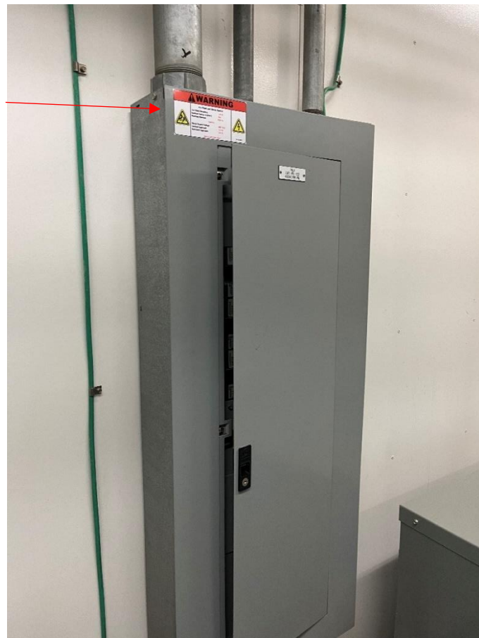
Figure 2: Electrical hazard door was open in the Cooling Tower I/O Building.
