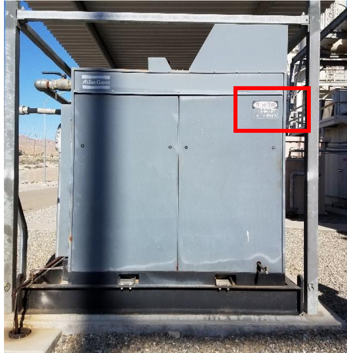
Figure 29: The Stage 1 air compressor has a faded/deteriorated danger sign.
