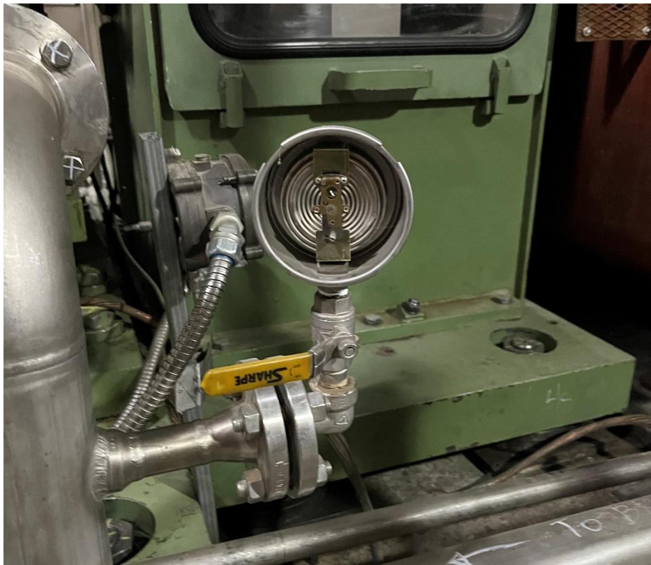
Figure 22: A gauge missing the dial, indicator and cover near Steam Turbine Generator.
