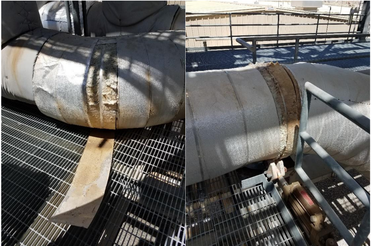
Figure 19: Piping insulation damaged/missing at second level of Unit 2.
