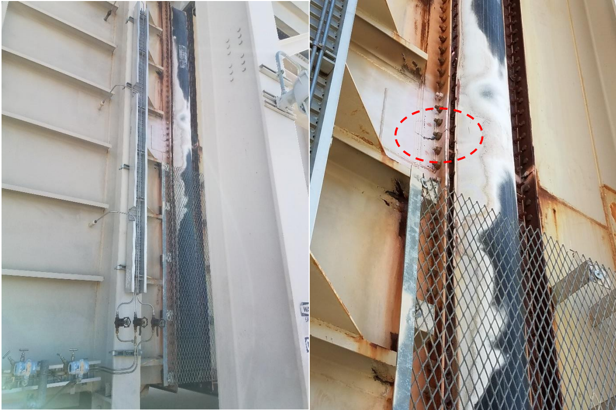
Figure 15: Heat damage and cracks along the fabric seal and cracking metal.
