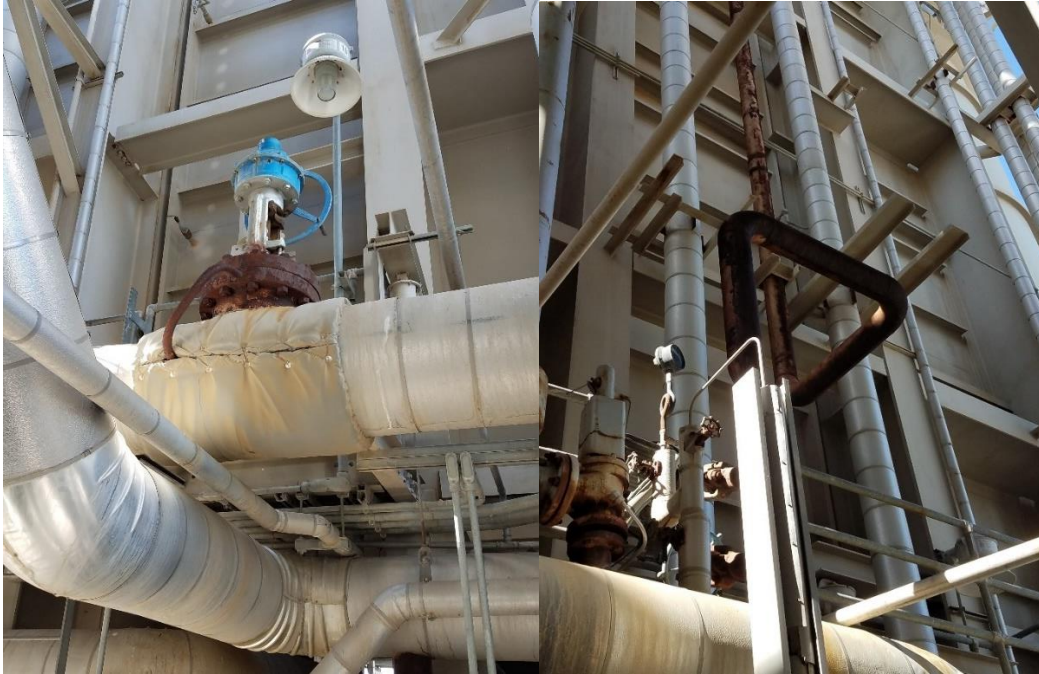
Figure 16: Flanges and piping at Unit 1 have moderate corrosion.
