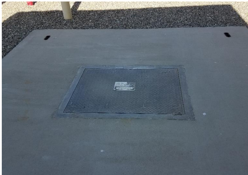
Figure 27: The manhole by the Stage 1 air compressor has a faded confined space sign.
