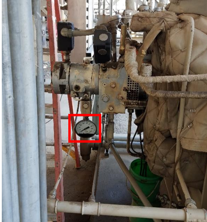
Figure 23: A gauge is filled with oil at boiler feed pump 201B.
