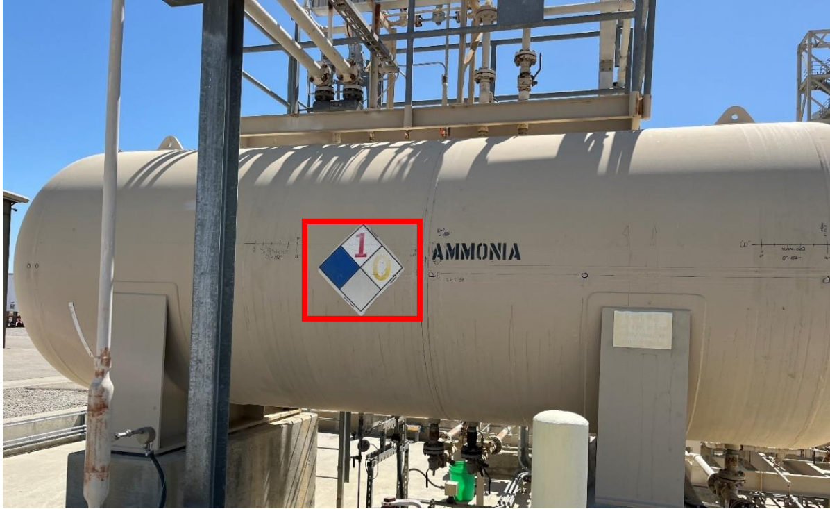
Figure 34: The Ammonia tank has a faded NFPA hazard diamond
