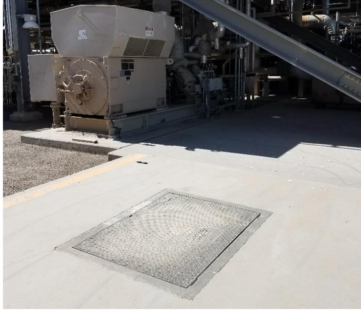
Figure 28: The manhole by Boiler Feed Pump 101A is missing a confined space sign.
