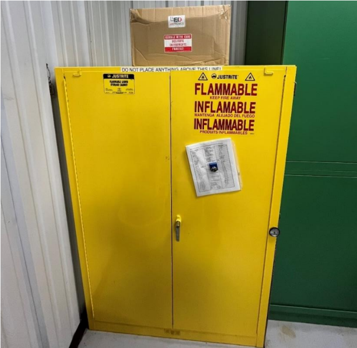
Figure 13: Flammable material cabinet has cardboard stored on top.
