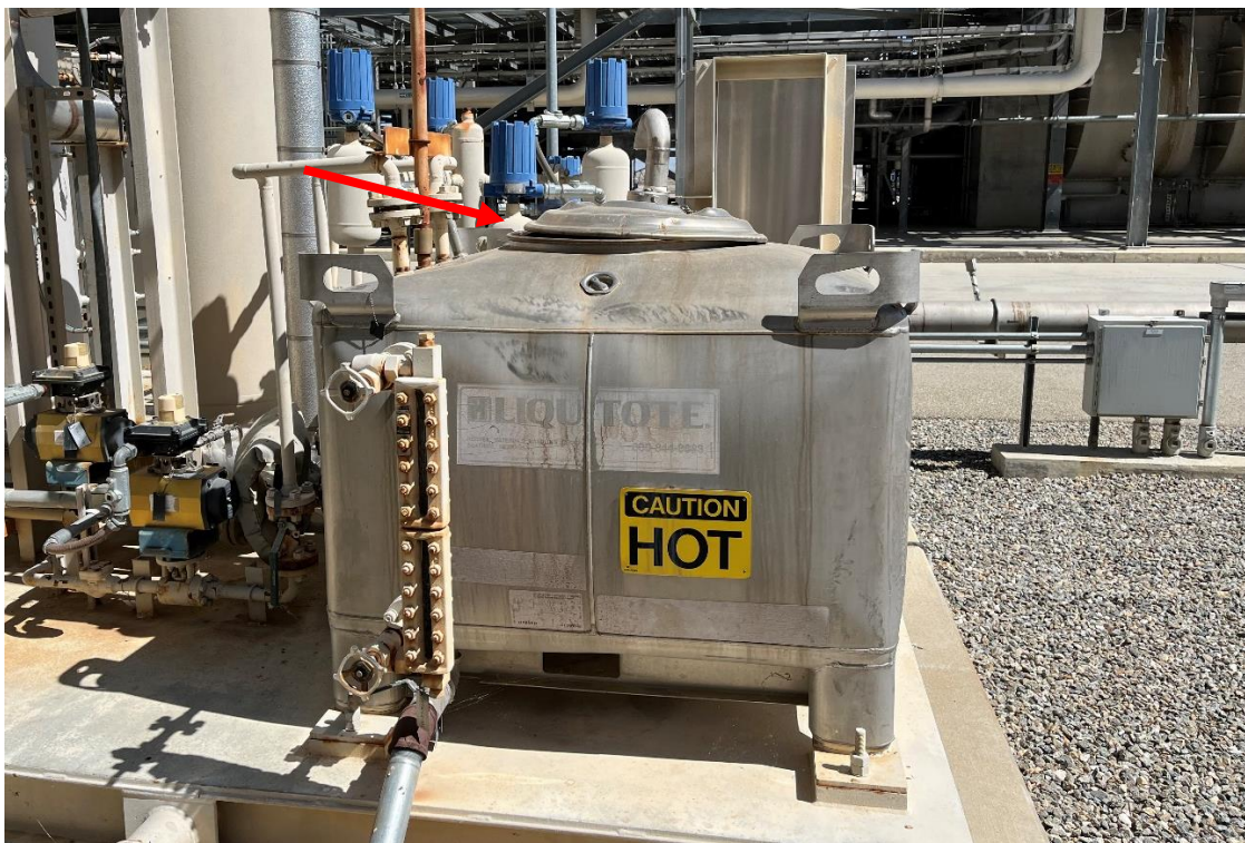
Figure 26: Lid ajar at the Fuel Heating Station
