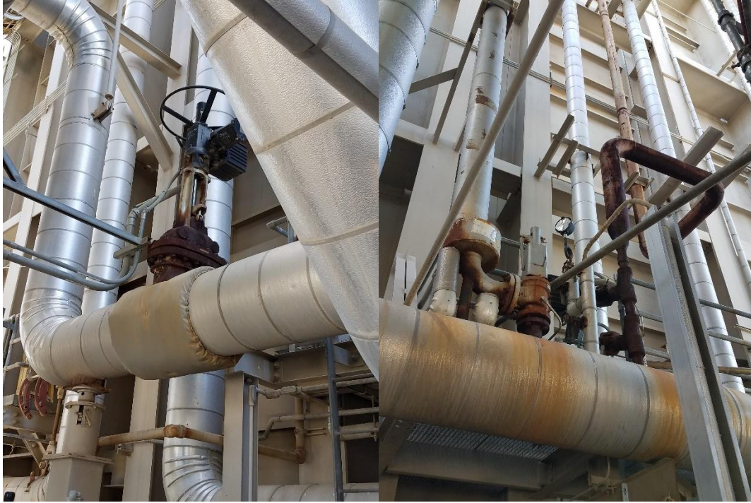
Figure 18: Flanges and piping at Unit 2 have moderate corrosion.
