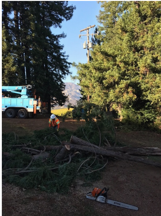
Figure 2. Near Calistoga, Sonoma County. Primary conductor damaged by fallen tree limb.
