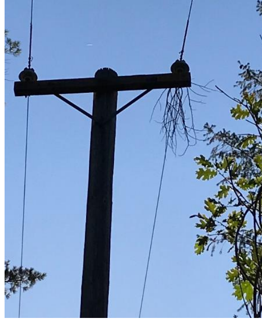
Figure 2 – Vegetation Debris Near 98 Gamble Rd, Oroville
