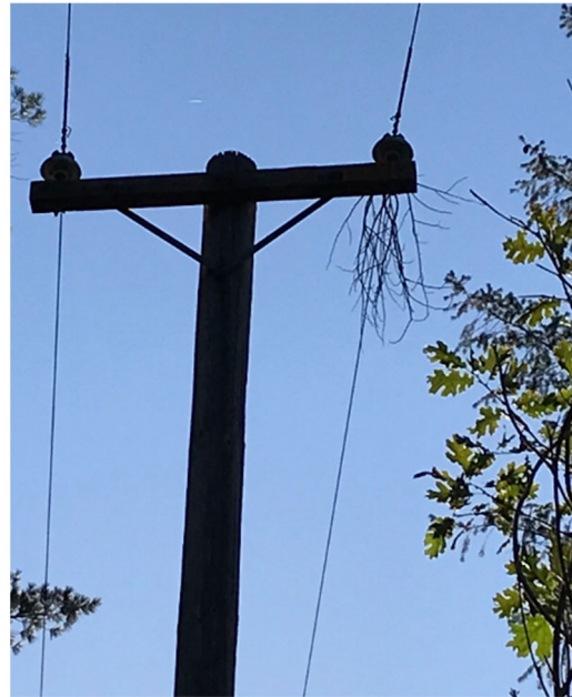
Figure 2 – Vegetation Debris Near 98 Gamble Rd, Oroville
