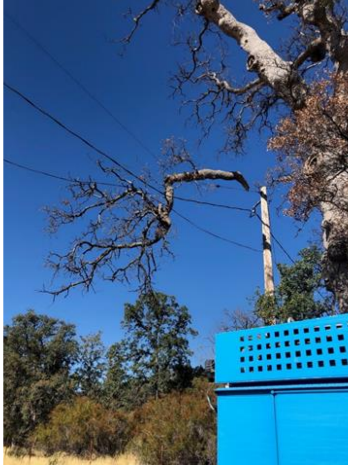
Figure 5 – In Stonyford, Colusa County Branch Flew Into Secondary Conductors
