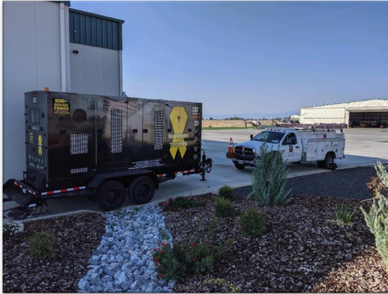
Figure 8 – Mobile Generation at PSPS-Critical Helicopter Hangar
