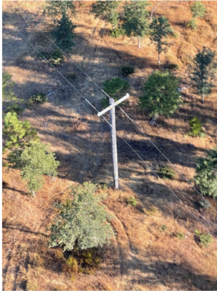
Figure 15: Vegetation-Damage in Shasta County – Broken tie wire
