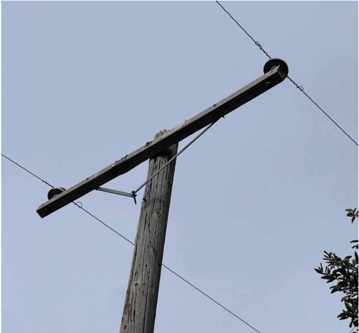
Figure 26 - Item #9 P166012 Crossarm Brace and Bolt Damage
