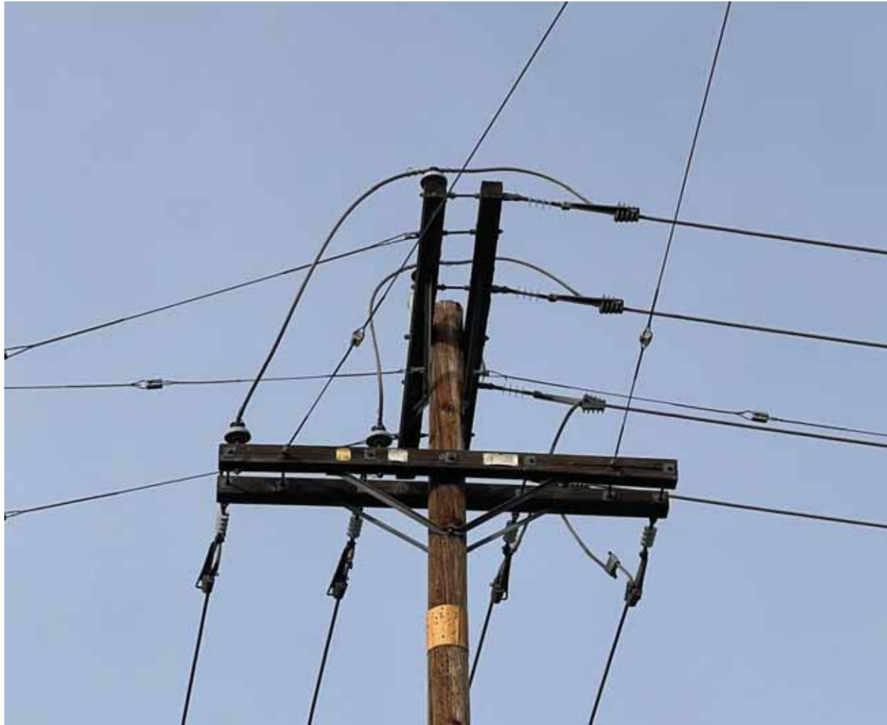
Figure 27 - Item #10 P179023 Damaged Crossarms
