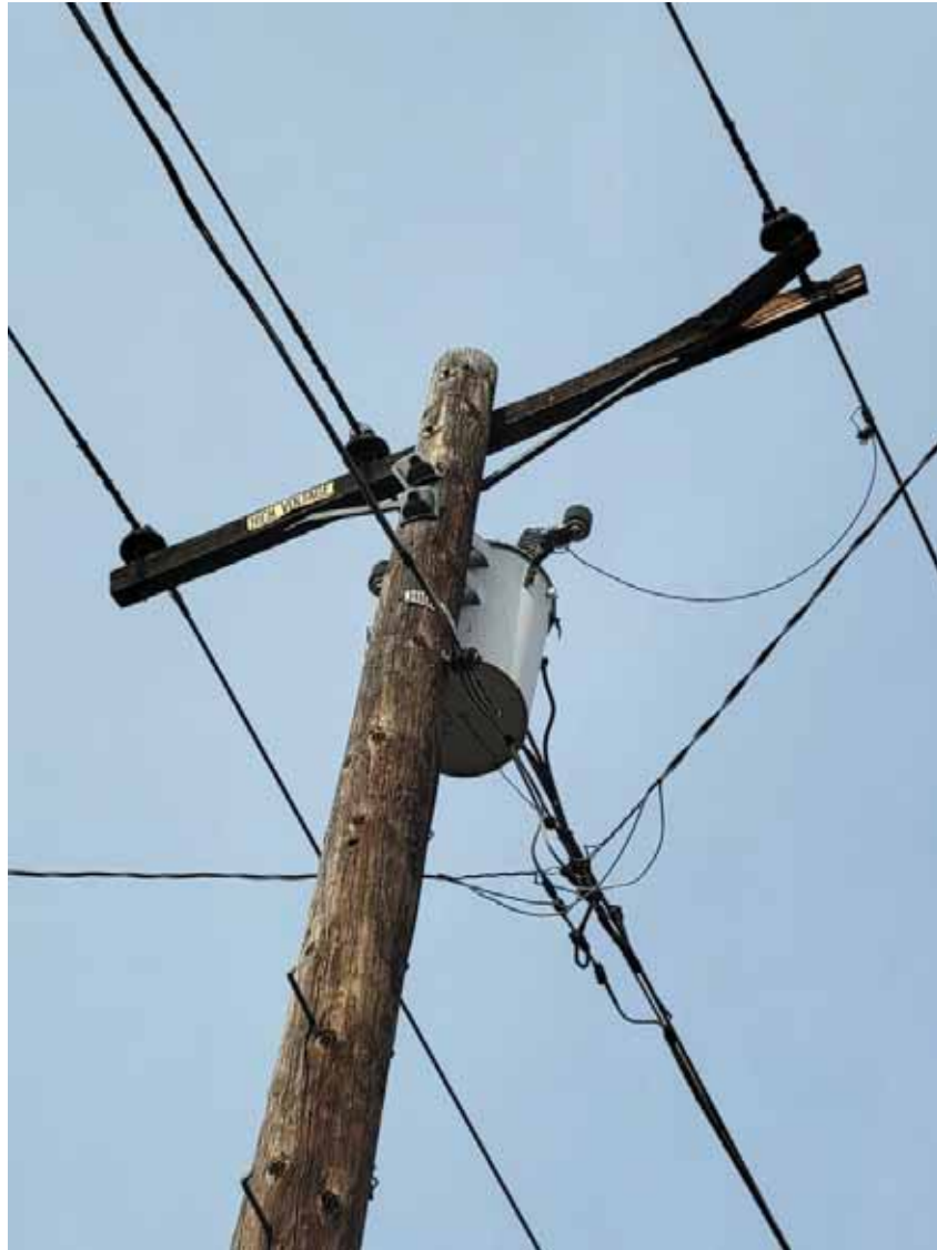
Figure 23 - Item #6 P516439 Damaged Crossarm
