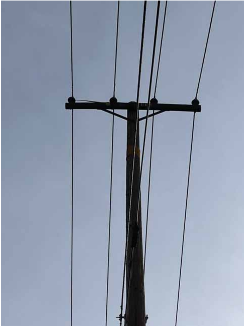
Figure 25 - Item #8 P78880 Damaged Crossarm
