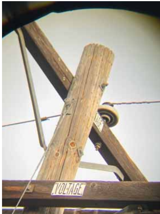
Figure 21 - Item #4 P119515 Damaged Crossarm
