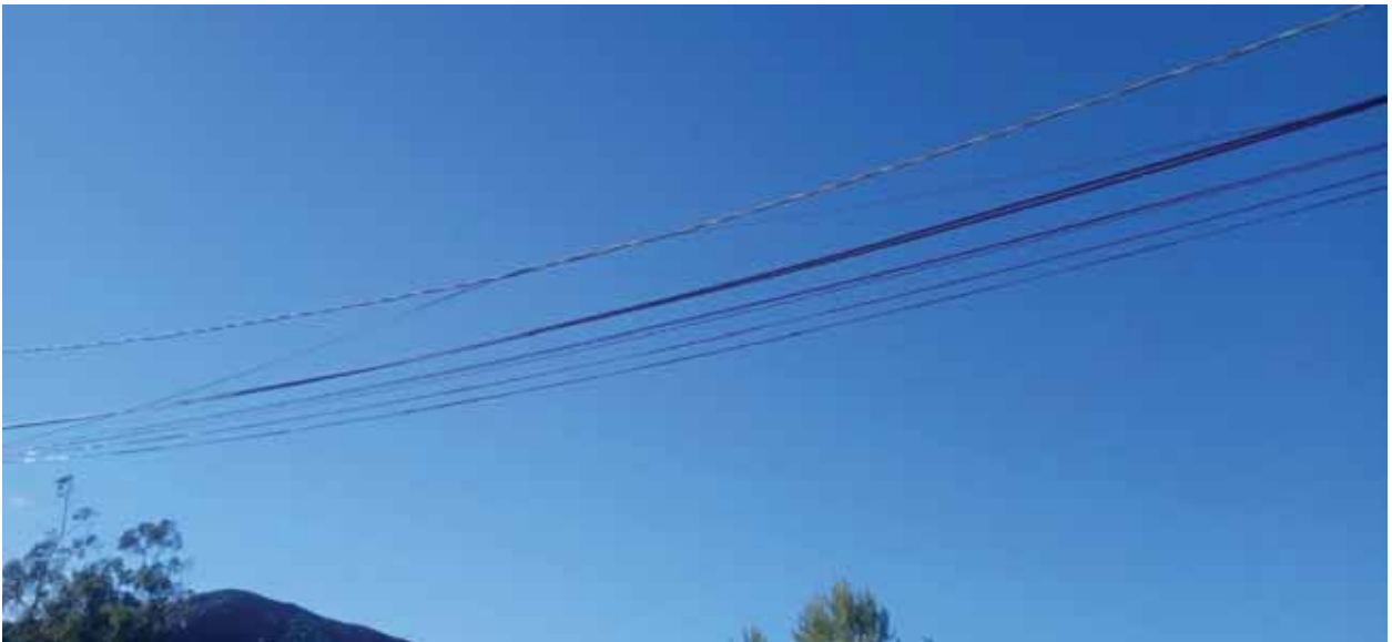
Figure 18 - Item #1 P710840 Telco Lashing
