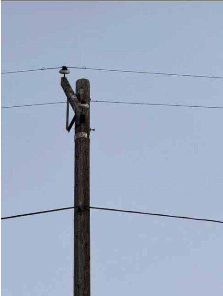
Figure 19 - Item #2 P376436 Crossarm Brace and Bolt Damage
