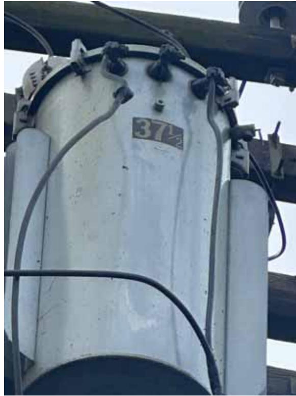
Figure 20 - Item #3 P213996 Leaking Transformer
