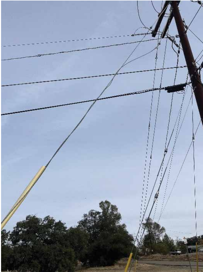
Figure 24 - Item #7 P78896 Broken Down Guy
