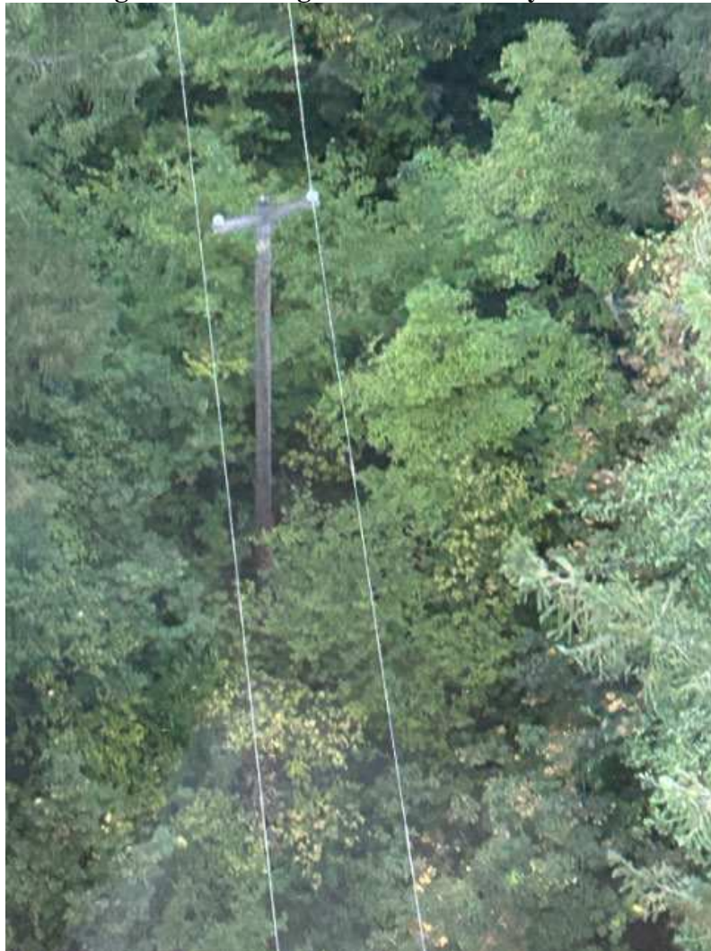
Figure 13: Vegetation-Damage in Shasta County – Broken Tie Wire
