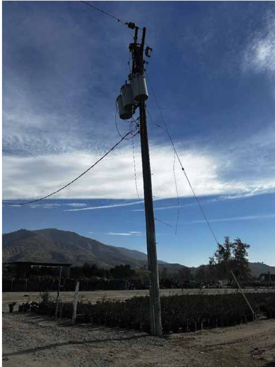
Figure 33 - Item #2 P106139 to P106138 Conductor Damage from Tree Branch
