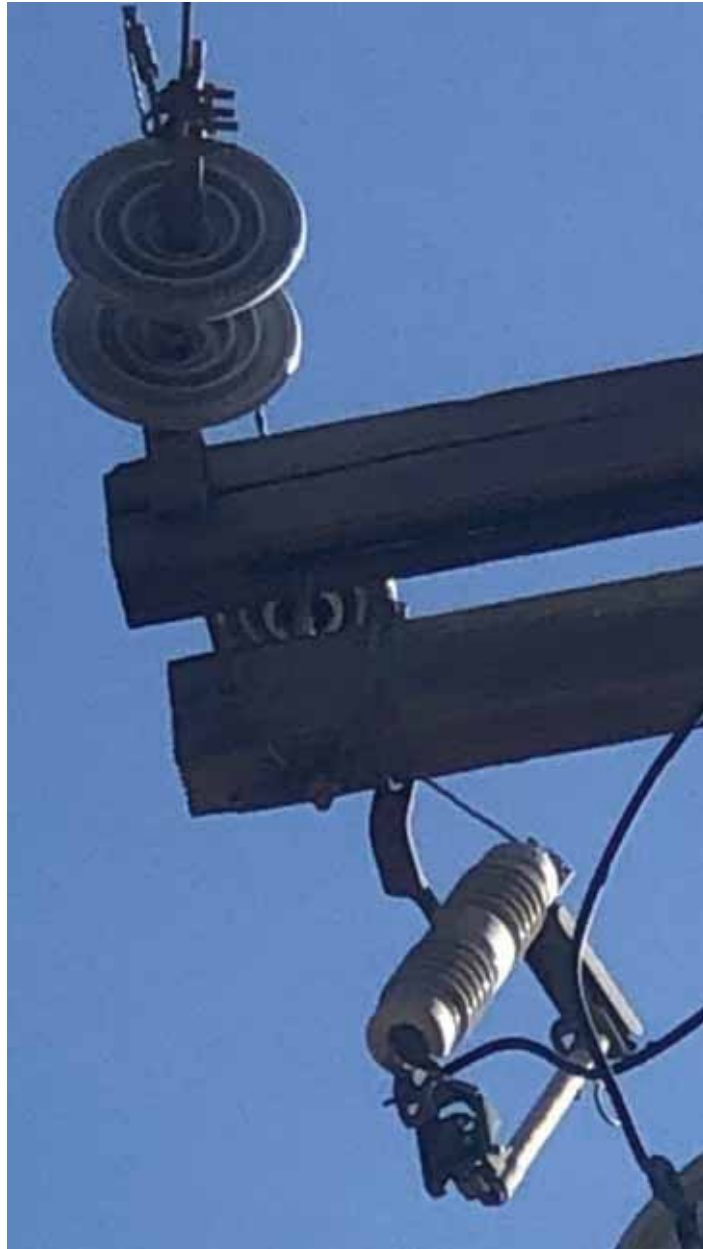
Figure 34 - Item #3 P228317 Damaged Crossarm
