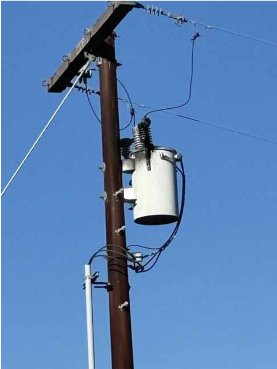
Figure 37 - Item #6 P716778 Transformer Damage
