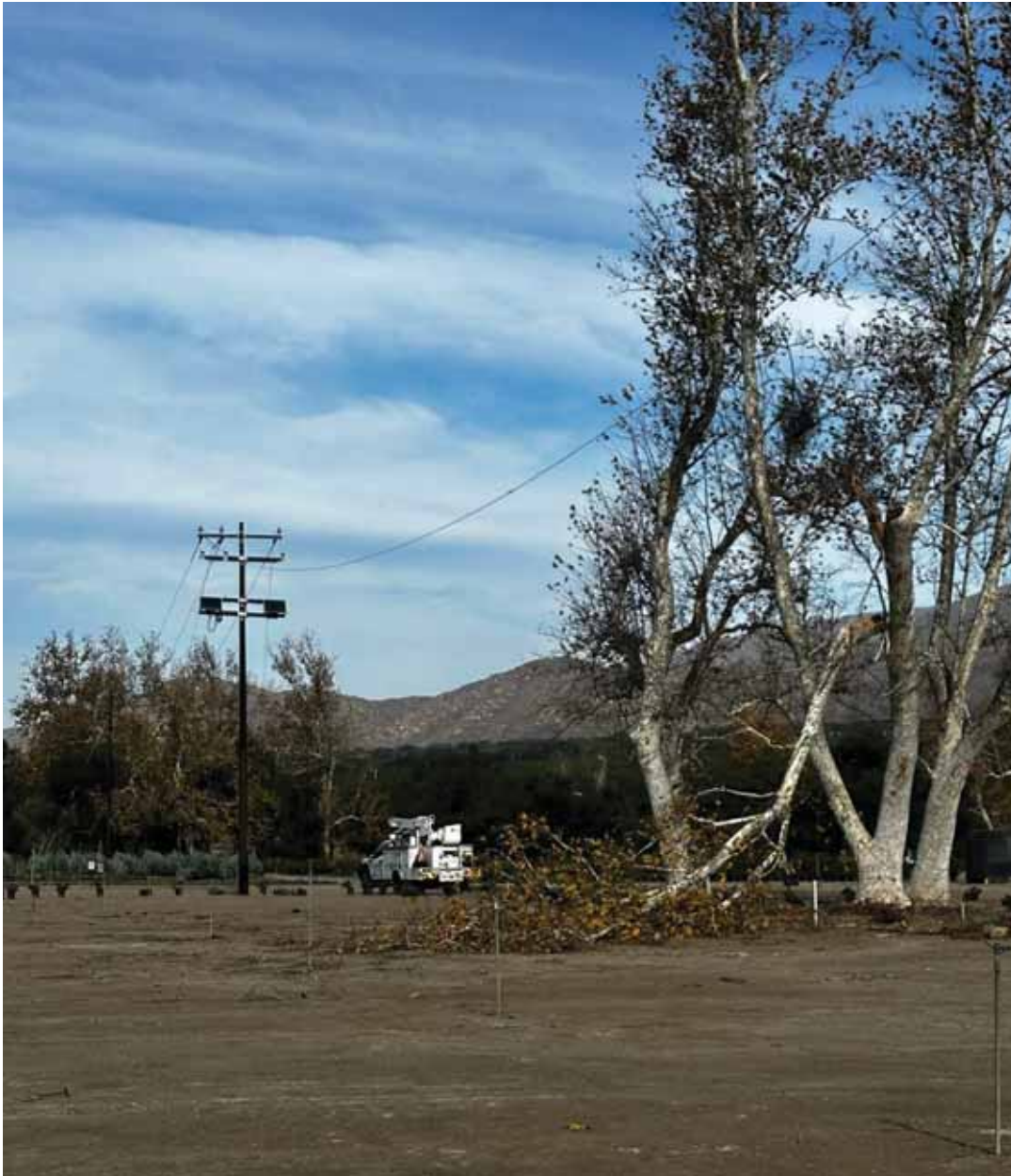
Figure 32 - Item #2 P106139 to P106138 Conductor Damage from Tree Branch
