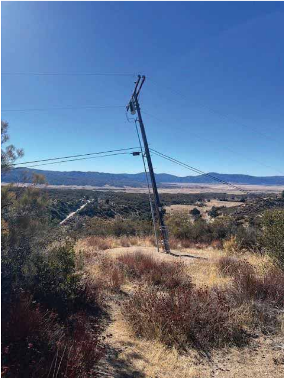
Figure 40 - Item #9 P410123 Leaning Pole
