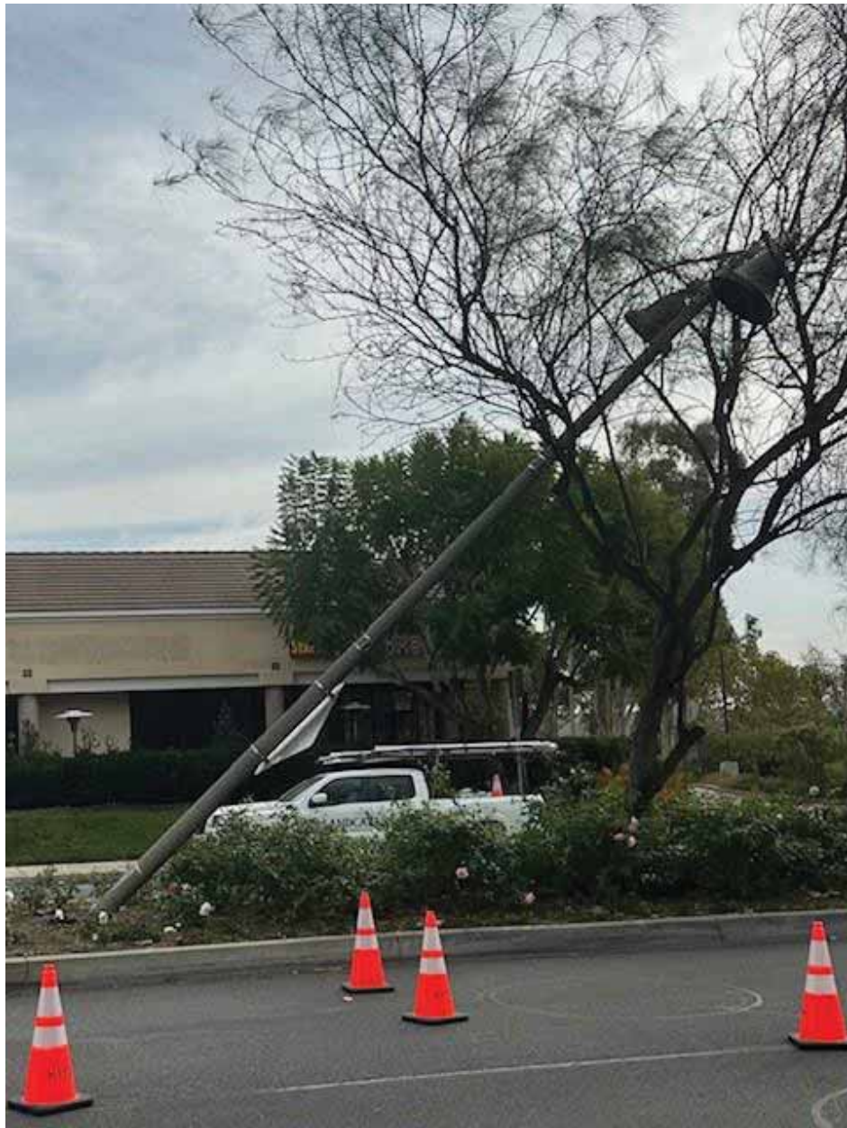
Figure 35 - Item #4 L121150 Streetlight Pole Fell Over
