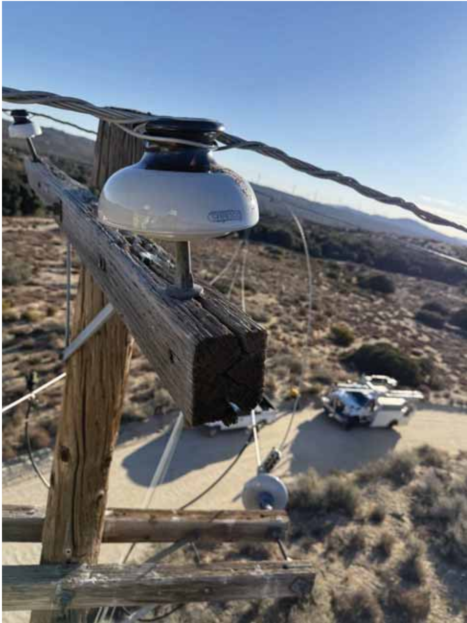
Figure 42 - Item #11 P46239 Damaged Crossarm
