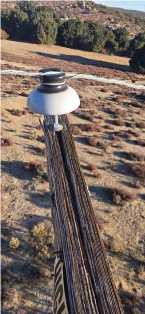
Figure 41 - Item #10 P46312 Damaged Crossarm
