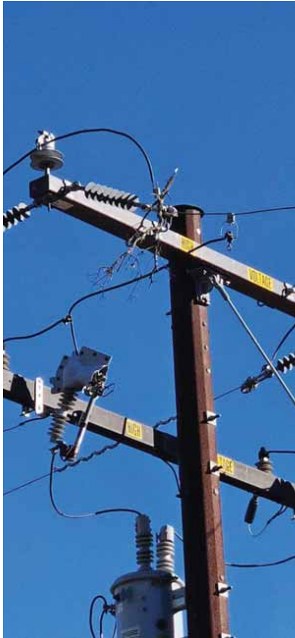
Figure 39 - Item #8 P711218 Tree Branch on Line
