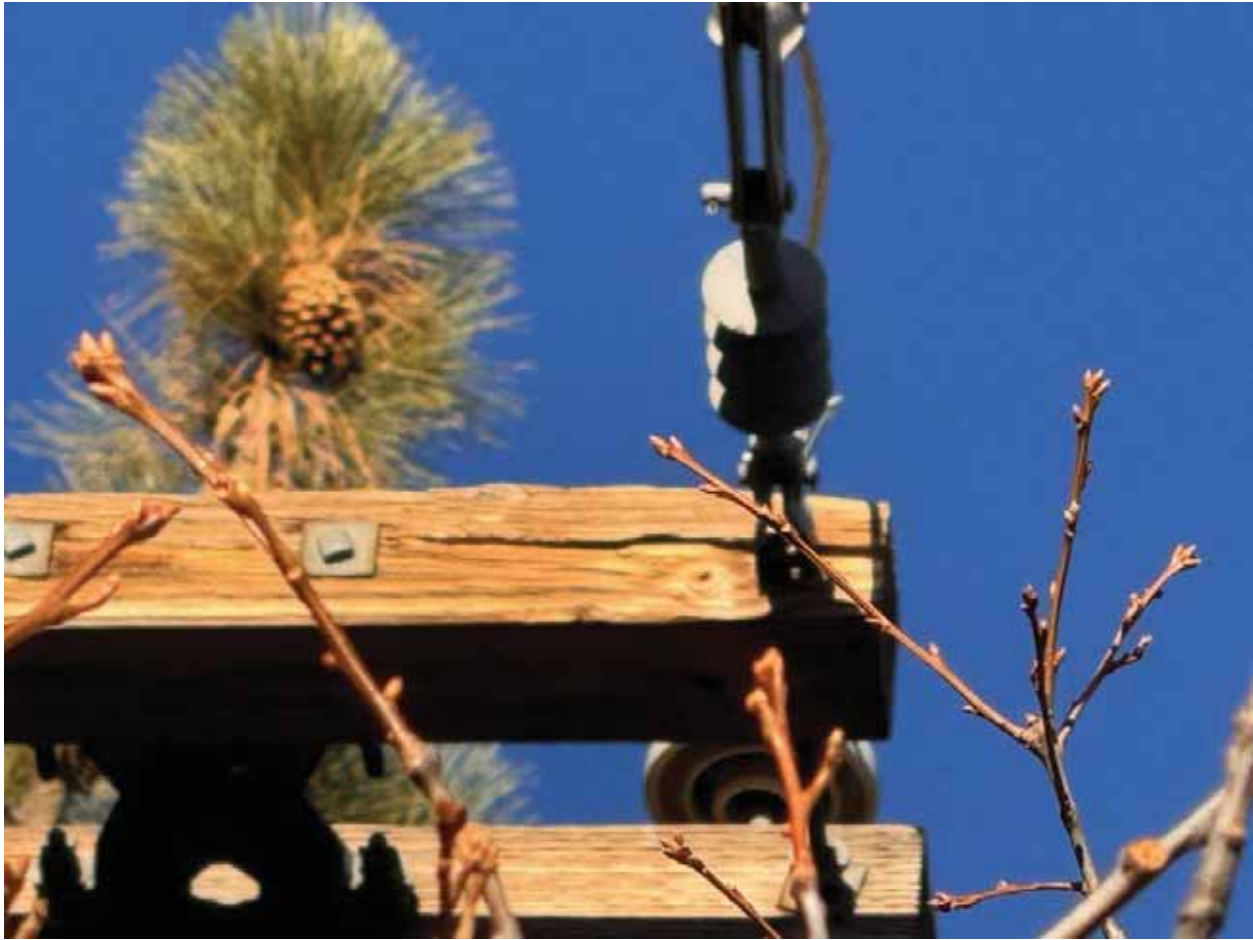
Figure 43 - Item #12 P233567 Damaged Crossarm
