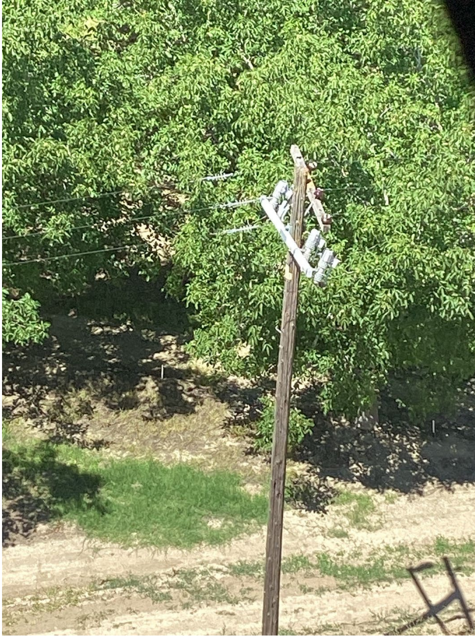
Figure 20: Wind Damage in Sutter County – Broken Insulator
