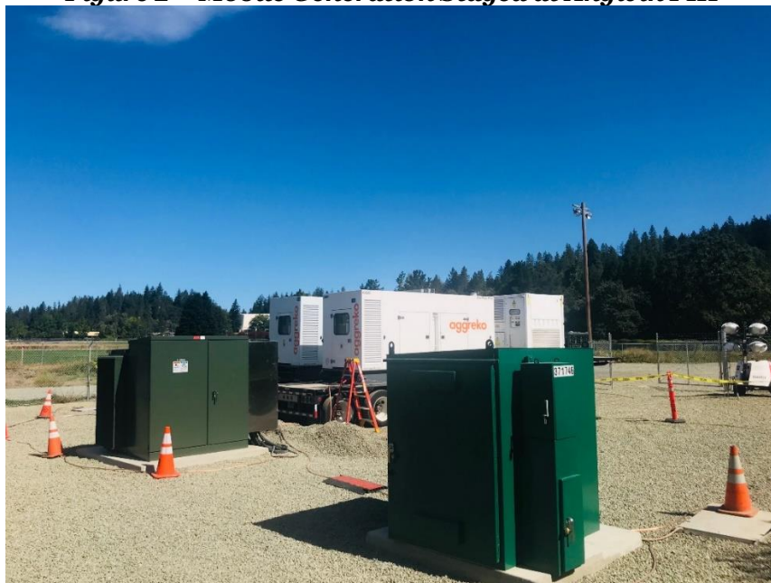
Figure 2 – Mobile Generation Staged at Angwin PIH
