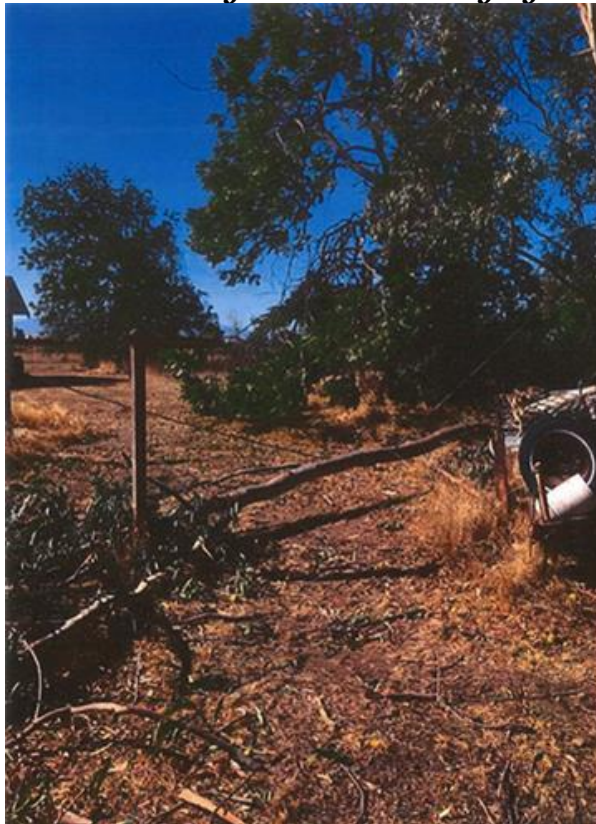
Figure 2 – In Artois, Glenn County Branch Fell Onto Secondary Conductors Bringing Down the Lines
