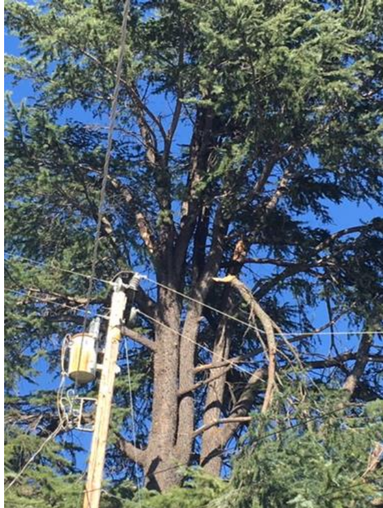
Figure 6 – In Red Bluff, Tehama County Branch Failed Into Primary Conductors
