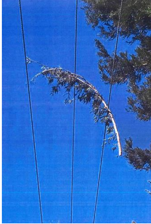
Figure 5 – In Cottonwood, Shasta County Branch Flew Into Primary Conductors
