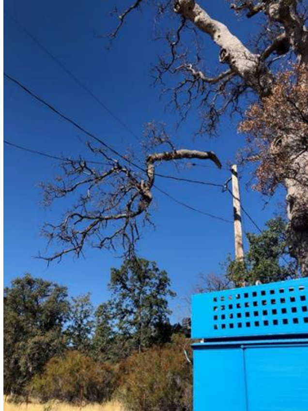
Figure 7 – In Stonyford, Colusa County Branch Flew Into Secondary Conductors
