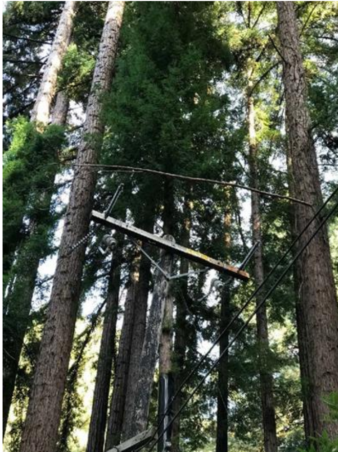
Figure 16 – In Boulder Creek, Santa Cruz County Branch in Contact Cross Phase Conductors
