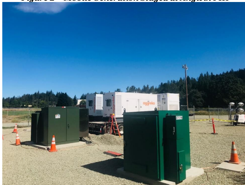
Figure 2 – Mobile Generation Staged at Angwin PIH
