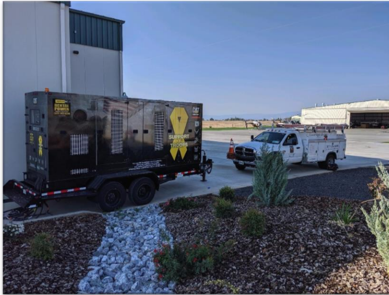
Figure 8 – Mobile Generation at PSPS-Critical Helicopter Hangar
