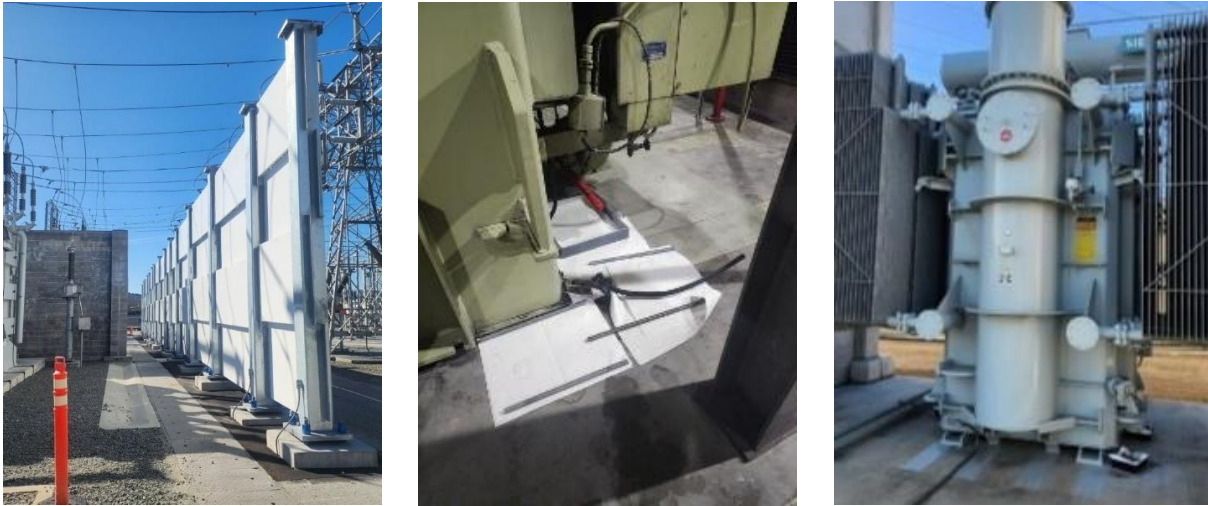
Figure 19: (Left) Ballistic wall; (Middle and Right) sample port oil leaks
