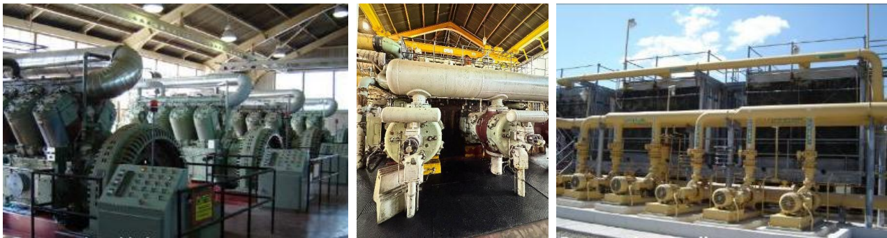
Figure 32: Photos of Compressor Station No.5
