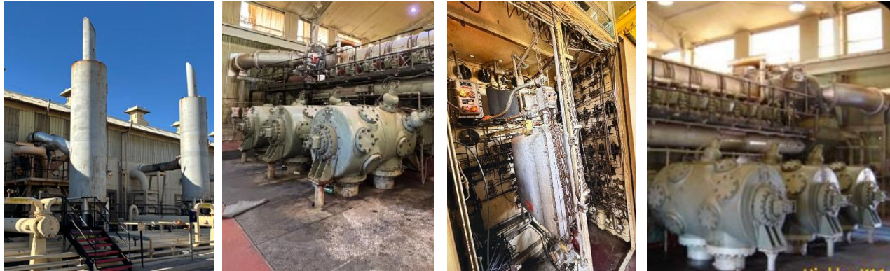
Figure 31: Photos of Compressor Station No.3
