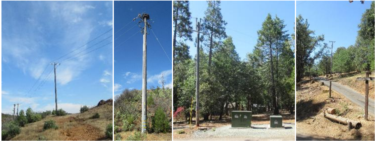
Figure 23: (Left to Right) FTI No trees observed; FTI Idle line; FTI Active underground conversion area tree removal in process; FTI Area conversion to underground tree removal and pruning completed.
