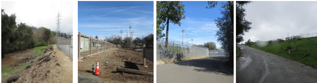
Figure 28: (Left to Right) Recent removal of vegetation to create buffer, erosion occurred; Vegetation buffer created wood framing on substation fence and wooden signage; Hardscape/Fencing, ladder fuels right side of entry drive; Tall vegetation removed, conversion to turf for buffer zone.
