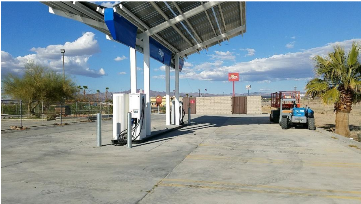
High Power-Charging station in Baker, CA, March 22,2018
