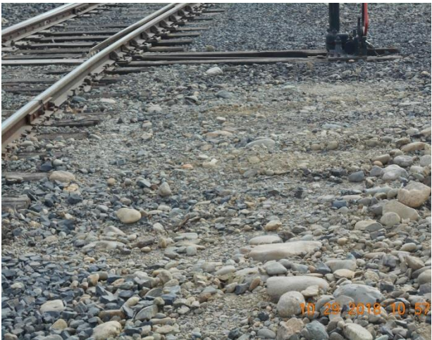
Walkway near derail switch with irregular surface
