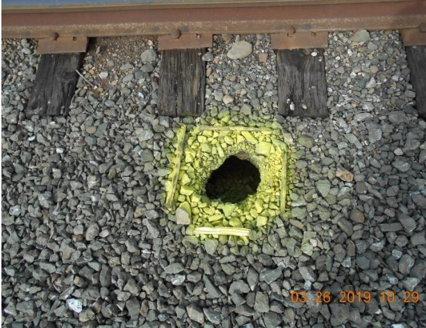
12 inch diameter by 12 inch deep hole in walkway
