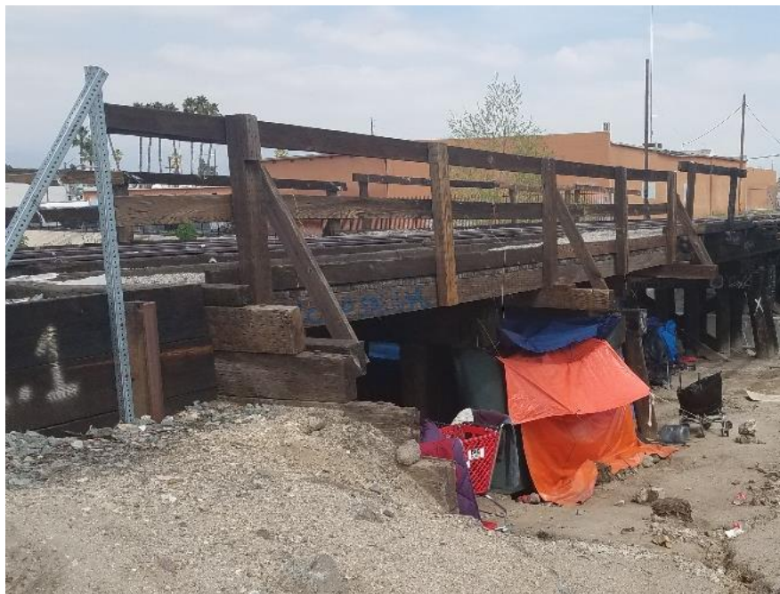
Homeless encampment under railroad bridge
