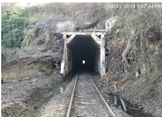
View of east entry to tunnel showing drainage ditches obstructed by debris
