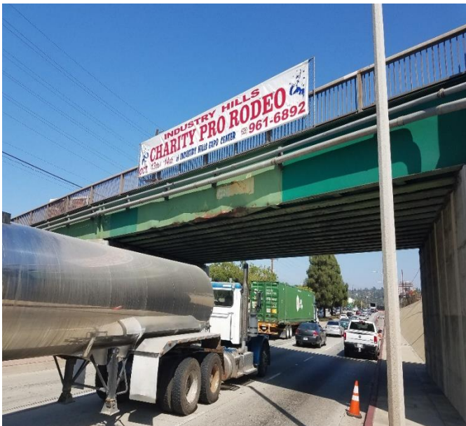
Damaged UPRR bridge, east side of Azusa Avenue, looking north
