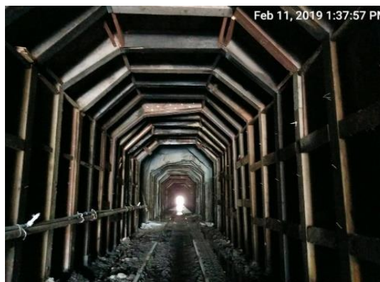
Mud inside tunnel caused by poor drainage
