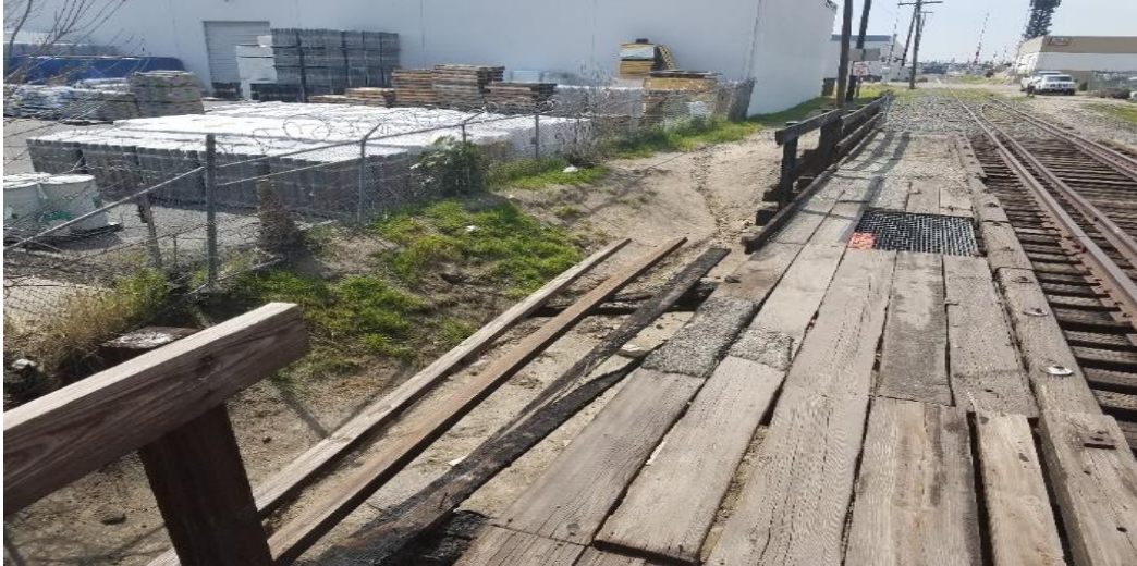
Missing handrail and deteriorated wooden walkway; violations of GO 118-A issued to railroad
