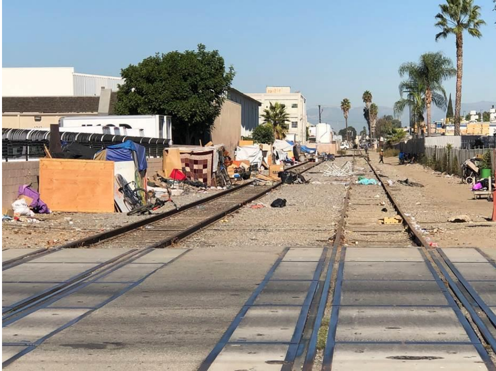
UPRR, Santa Ana - Costa Mesa industrial lead, Warner Avenue. Note debris on left track and proximity of structures to track.
