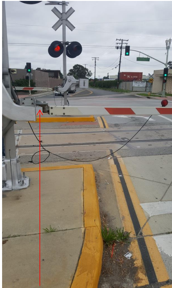
Unattached gate arm light wire; red arrow shows proper attachment point
