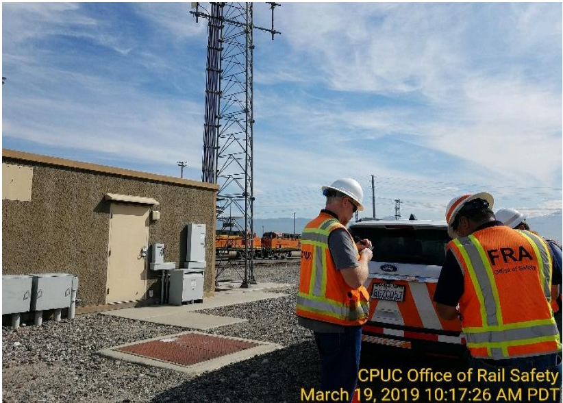
BNSF PTC wayside location observed by CPUC inspectors in conjunction with an FRA inspector
