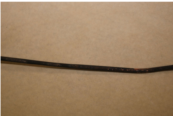
Figure 6: Damaged east conductor.
