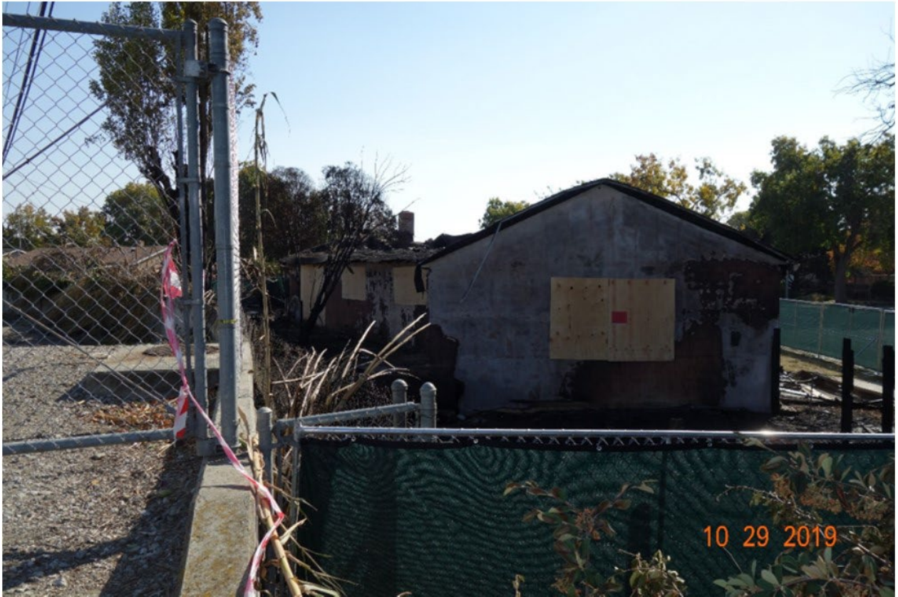
Figure 2: Fire 2 on South Side of Marylinn Drive, Milpitas, CA
