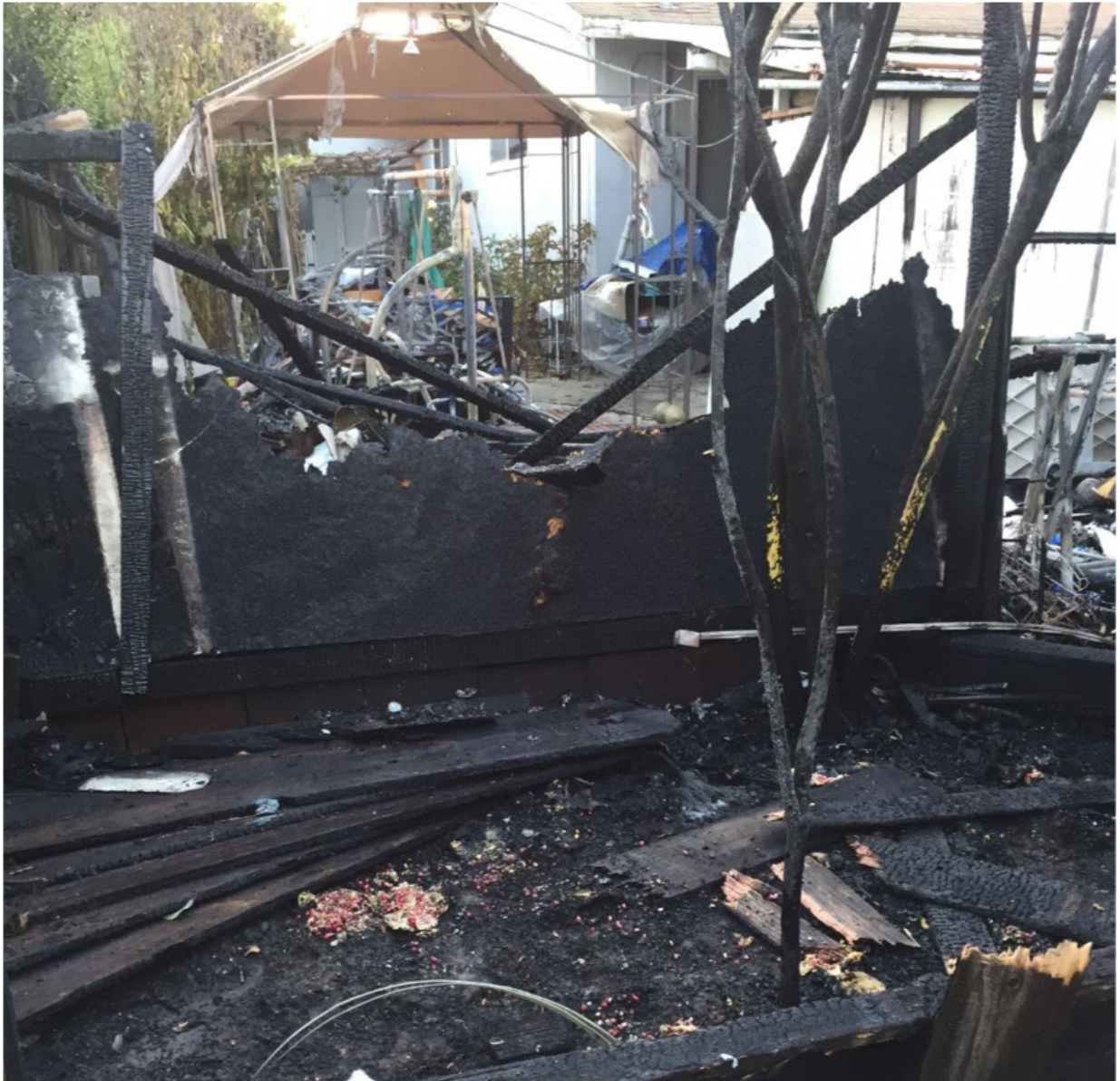
Figure 3: Fire 3 at 235 Casper Street
