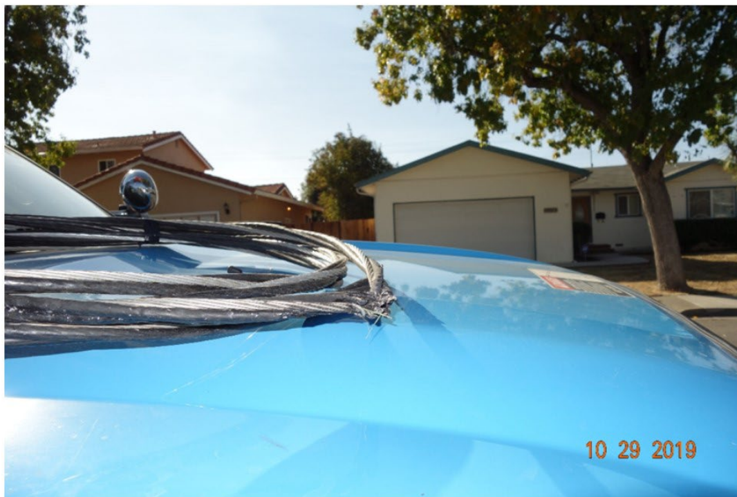
Figure 7: Damaged Service Drop
