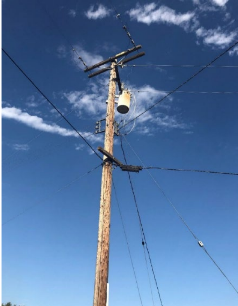
Figure 6. Photo showing the transformer pole. No work was performed on this pole (Source: PG&E).
