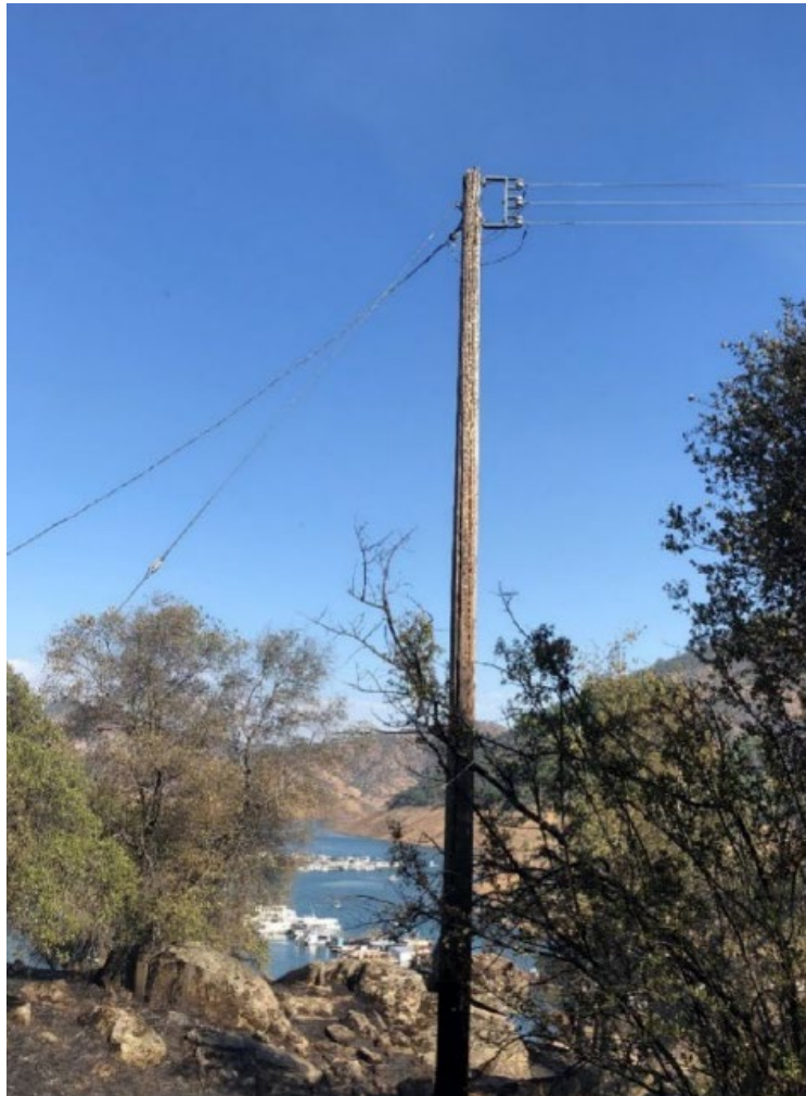
Figure 4. Photo showing the 35-foot secondary pole with vertical rack configuration. PG&E replaced this pole with a new 40-foot pole and triplex with a horizontal configuration (Source: PG&E).
