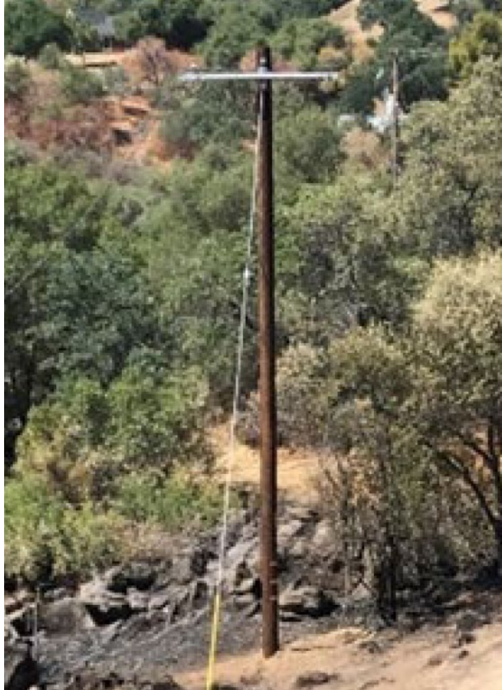
Figure 5. Photo showing the new 40-foot replacement pole and triplex with a horizontal configuration (Source: PG&E).
