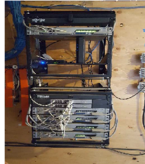
Figure 11: CASF Public Housing Account project Housing Authority of the County of Kern – Green Gardens MDF room.
