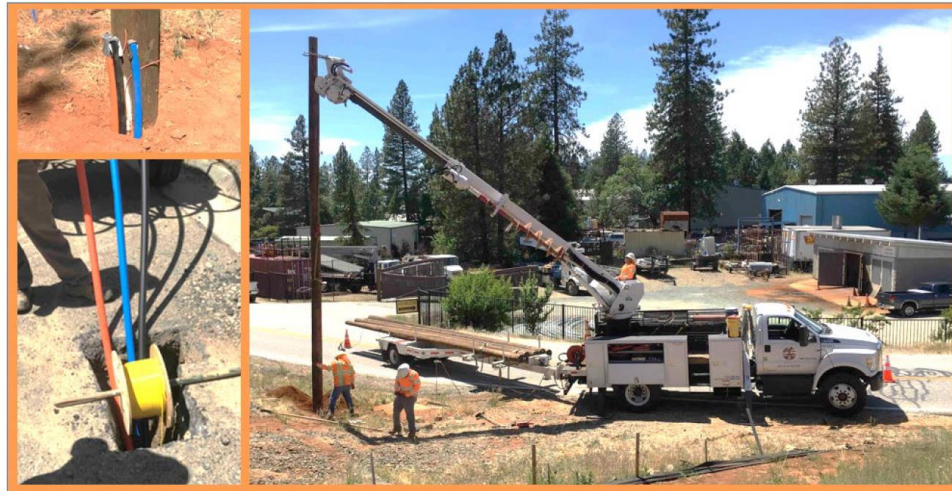
Figure 4: Deployment of Race Telecommunications' CASF fiber-to-the-premises Bright Fiber project in Nevada County
